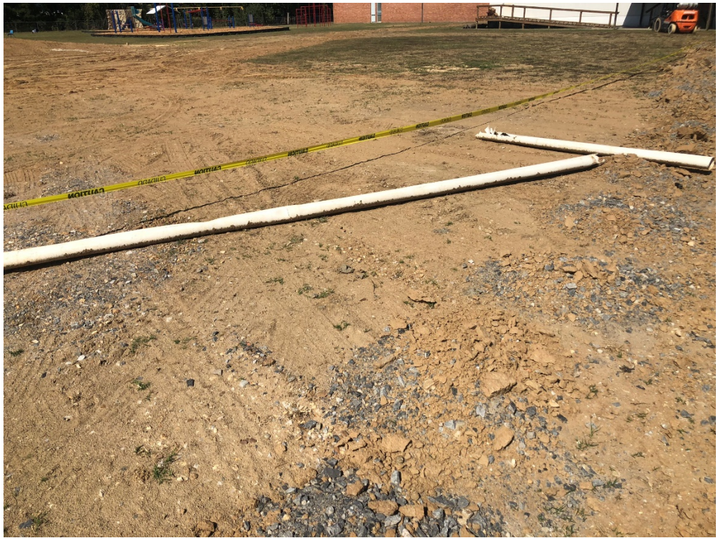
Figure 9 – Undisposed Excavated Drain Pipe
