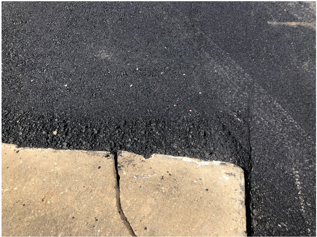
Figure 3 – Unfinished Paving at South Corner and Existing Sidewalk
