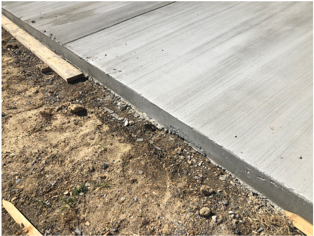
Figure 11 – Undisposed Formwork at Dumpster Slab
