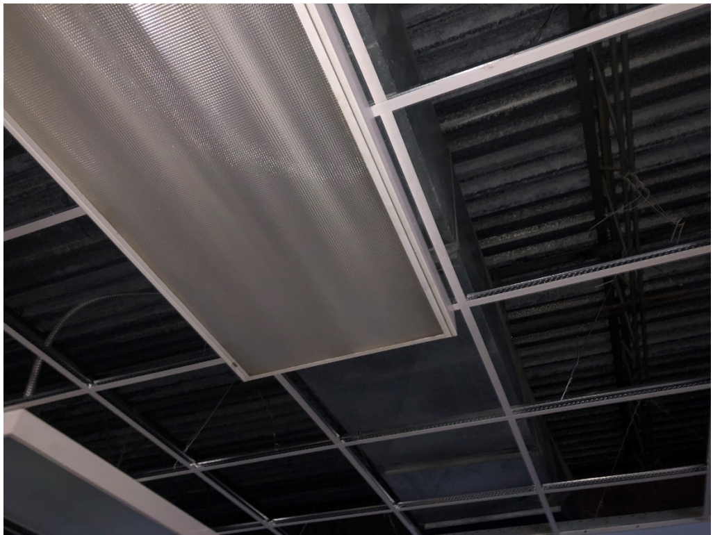
Figure 30 – Misaligned light with Framework
