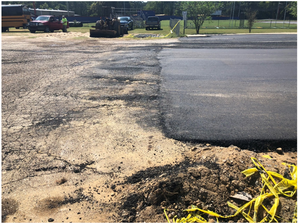
Figure 13 – New Paving Even with Existing Paving
