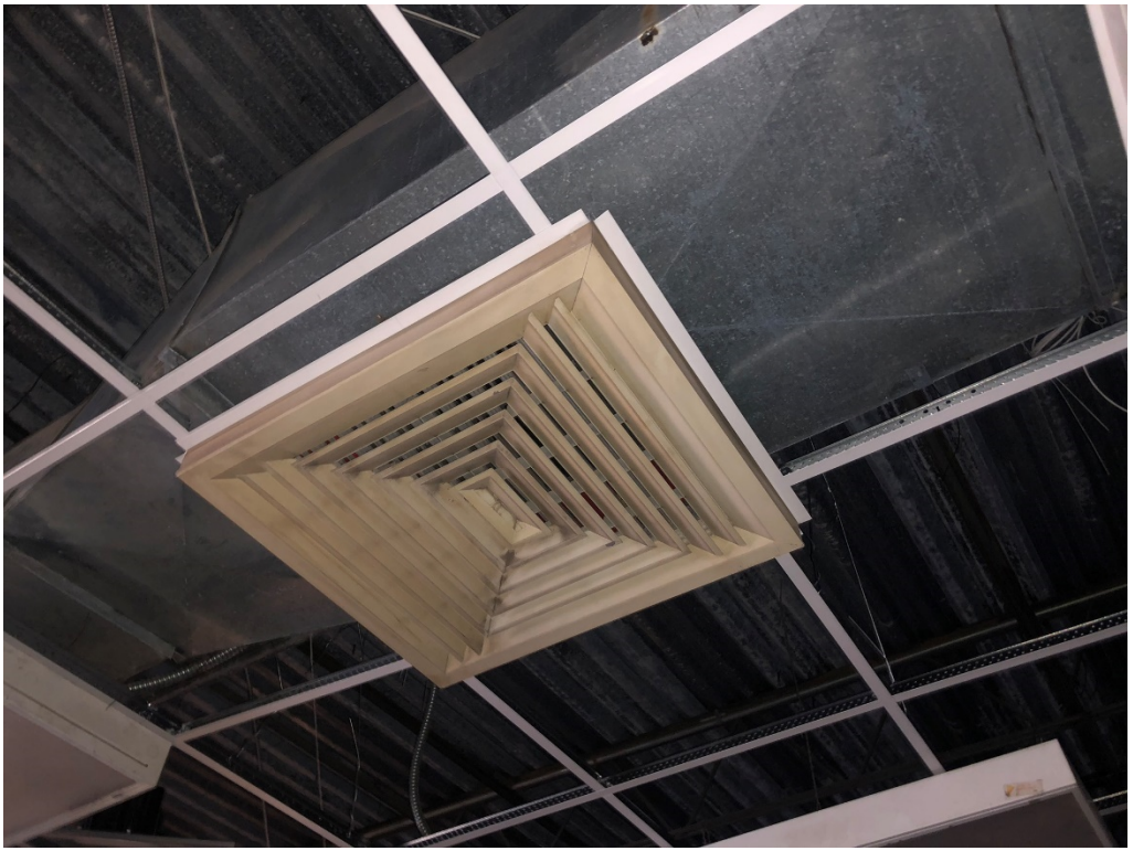
Figure 31 – Unfinished Grid Corners
