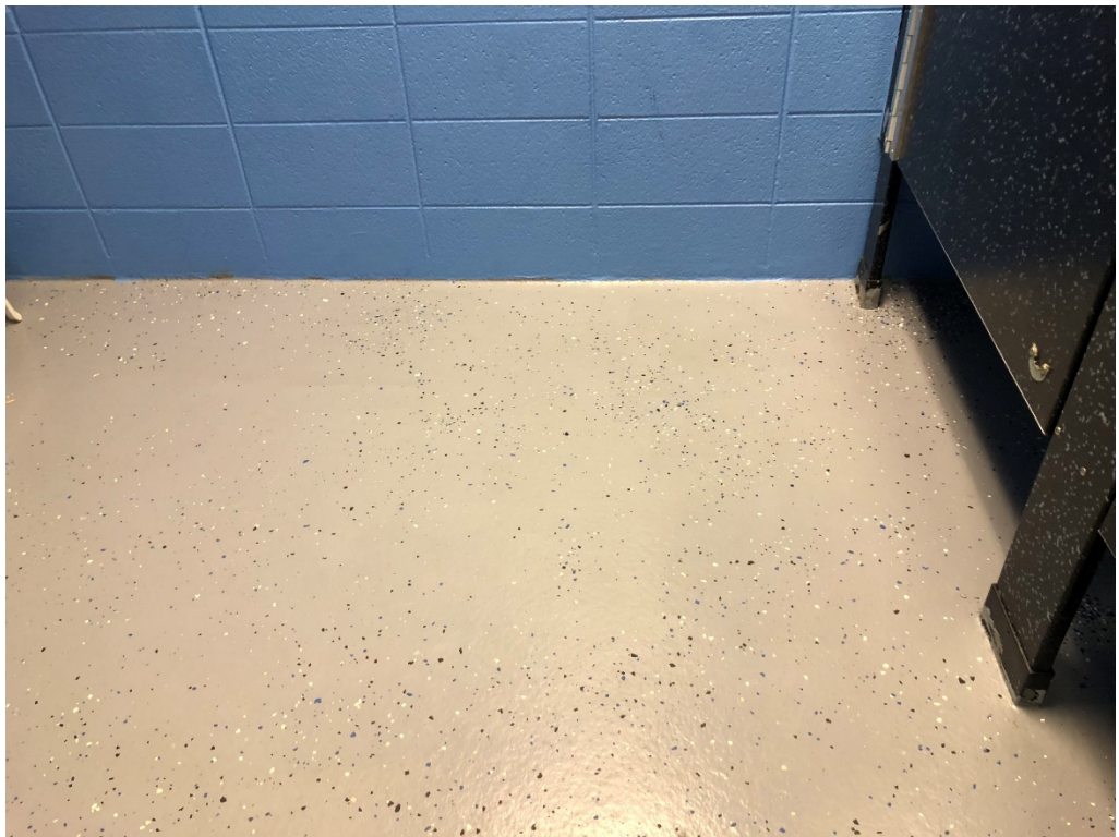
Figure 18 – Previously Painted Bathroom
