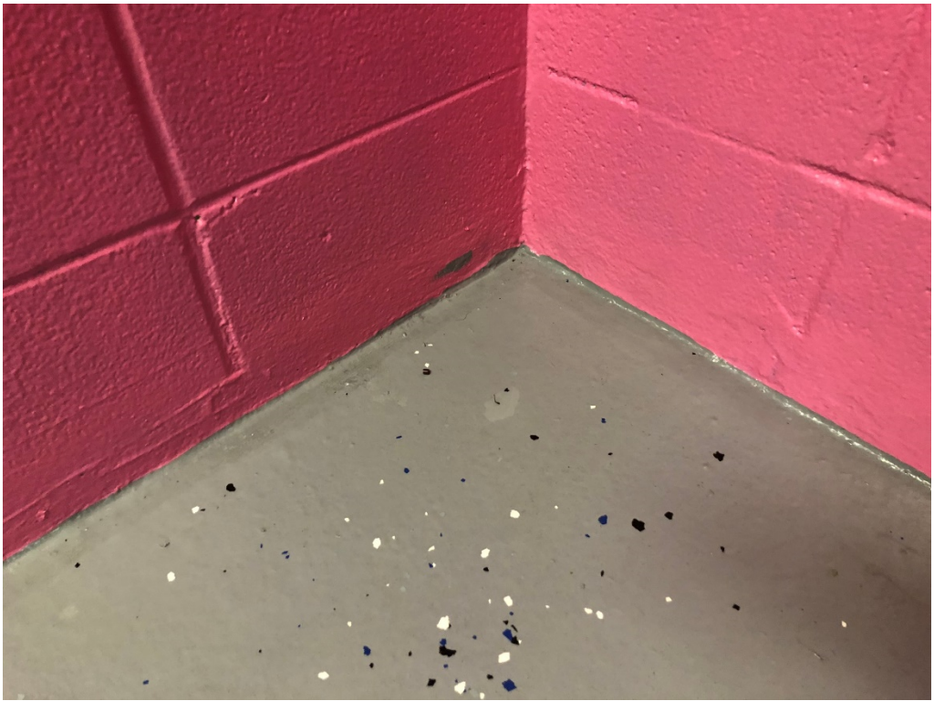
Figure 25 – Paint on Wall (Typical)
