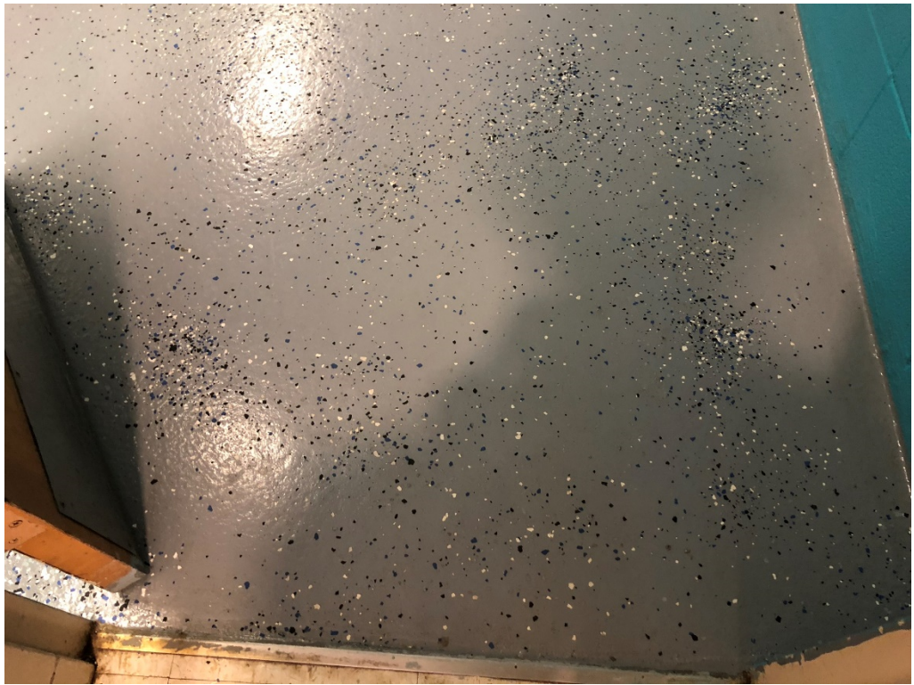
Figure 15 – Previously Painted Bathroom
