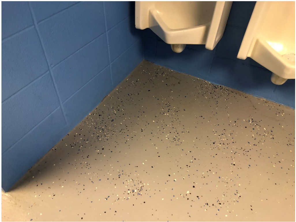
Figure 17 – Previously Painted Bathroom
