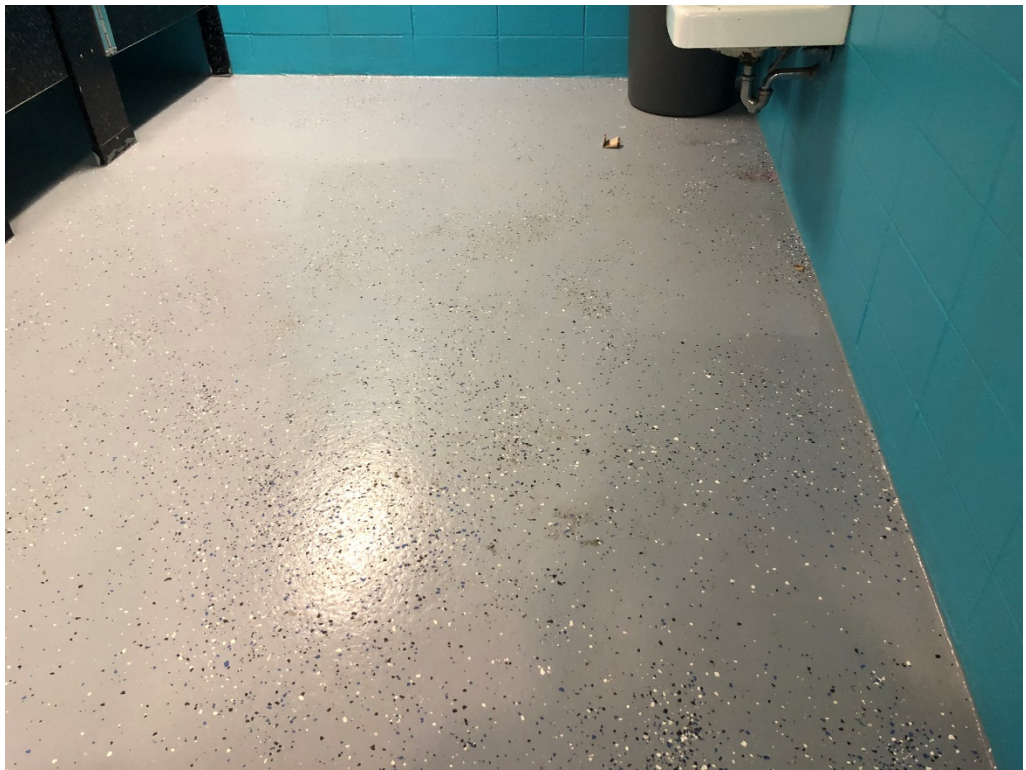
Figure 14 – Previously Painted Bathroom
