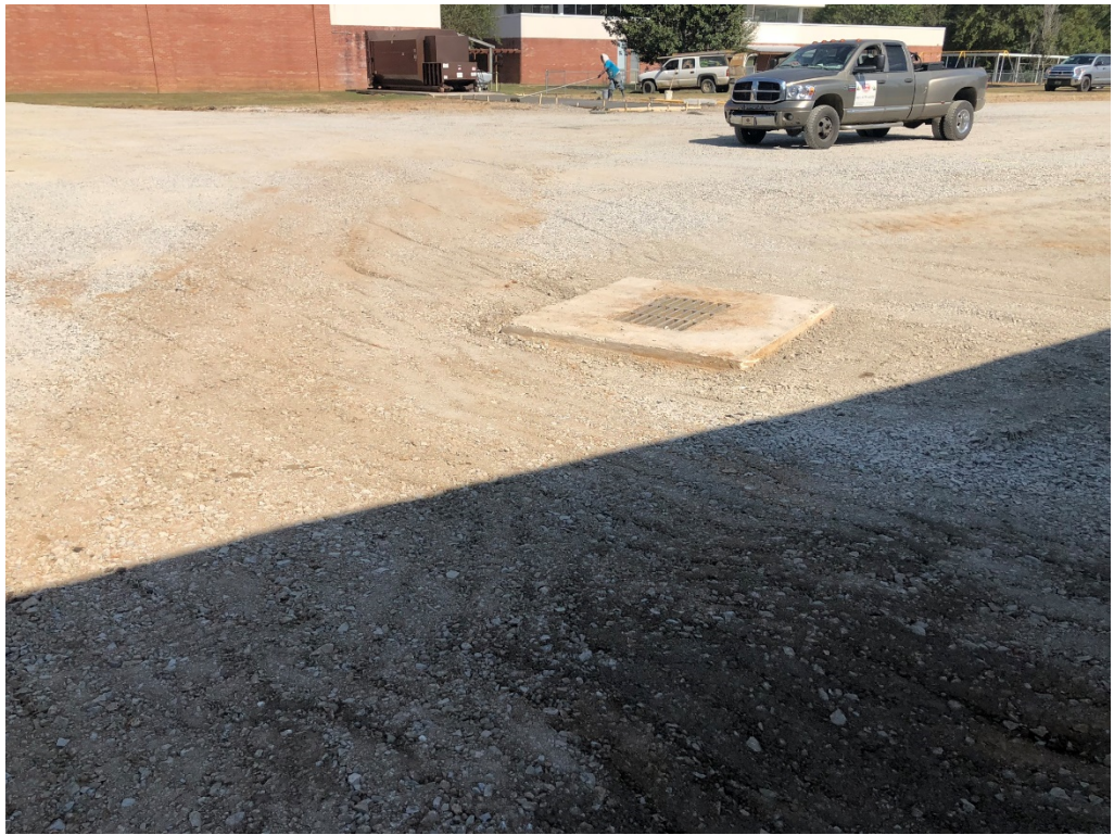
Figure 5 – West Side of Parking (area that sewer was Damaged and Replaced)
