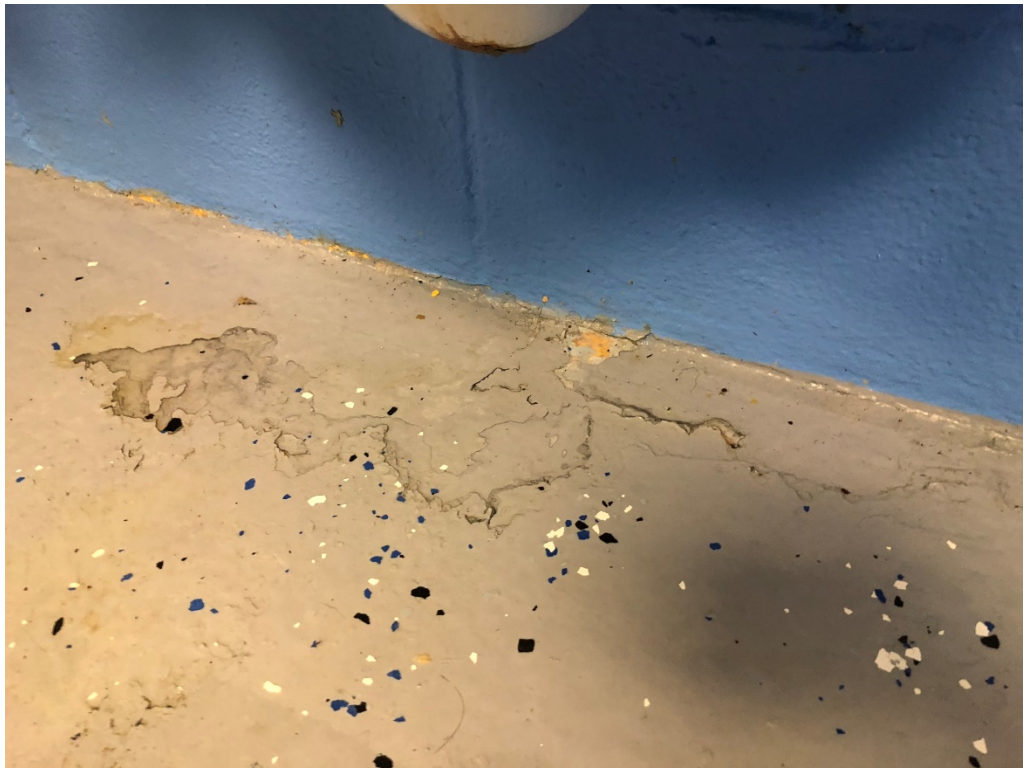
Figure 23 – Failed Paint from Previous Work (NOT Typical)
