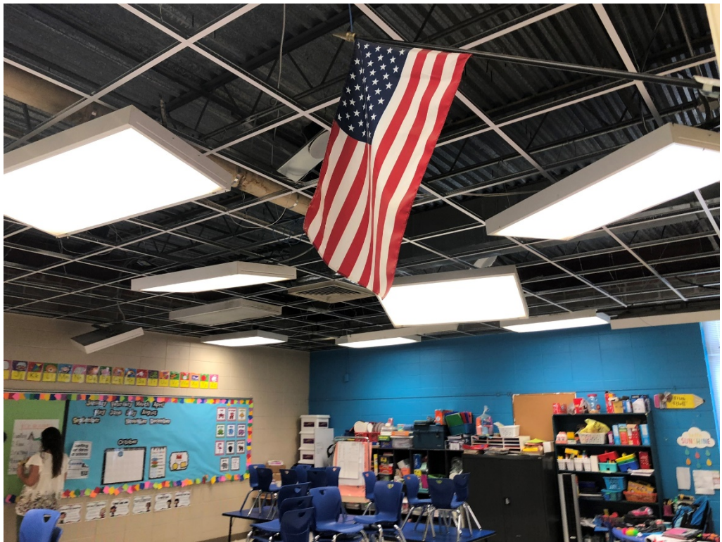
Figure 20 – Classrooms with Removed Tile
