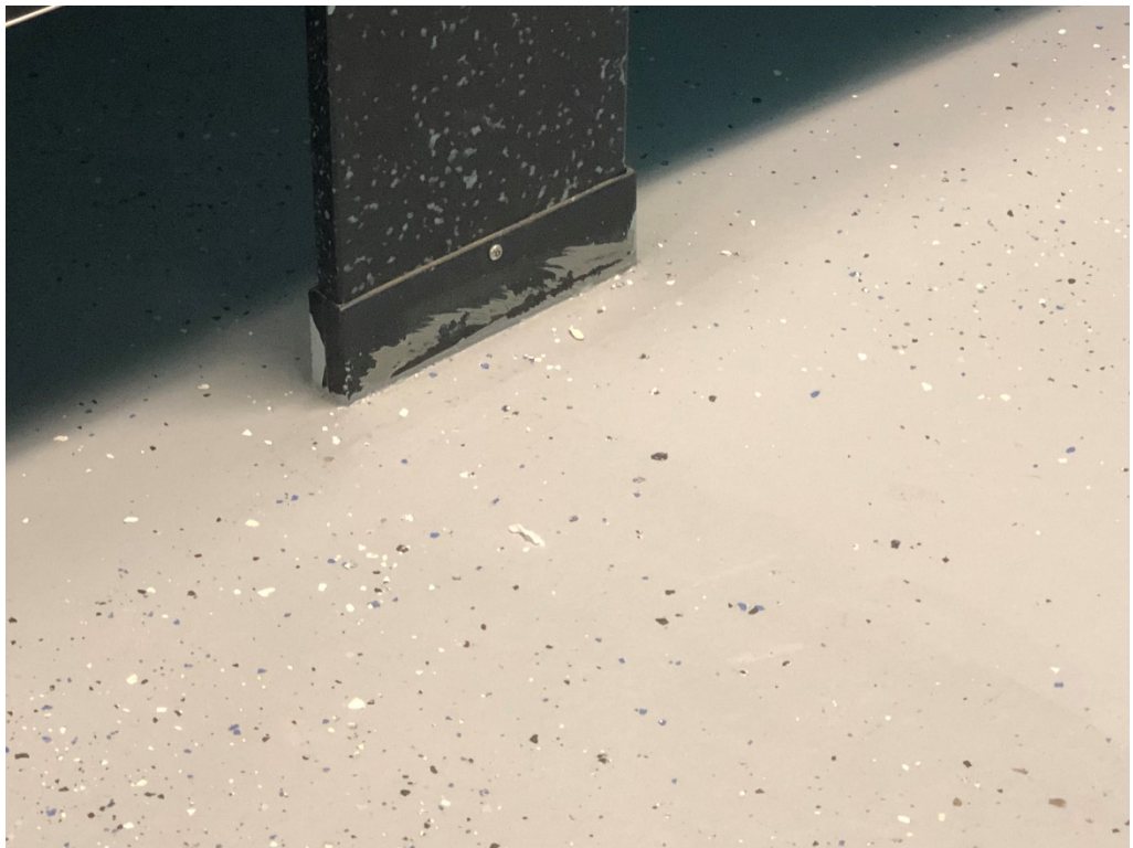
Figure 16 – Paint Noted on Toilet Partitions (Typical)
