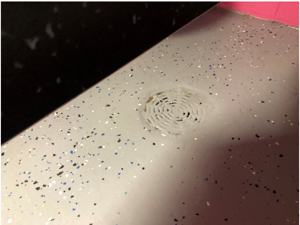
Figure 26 – Floor Drains More than 50% Blocked By Previous Work (Typical)
