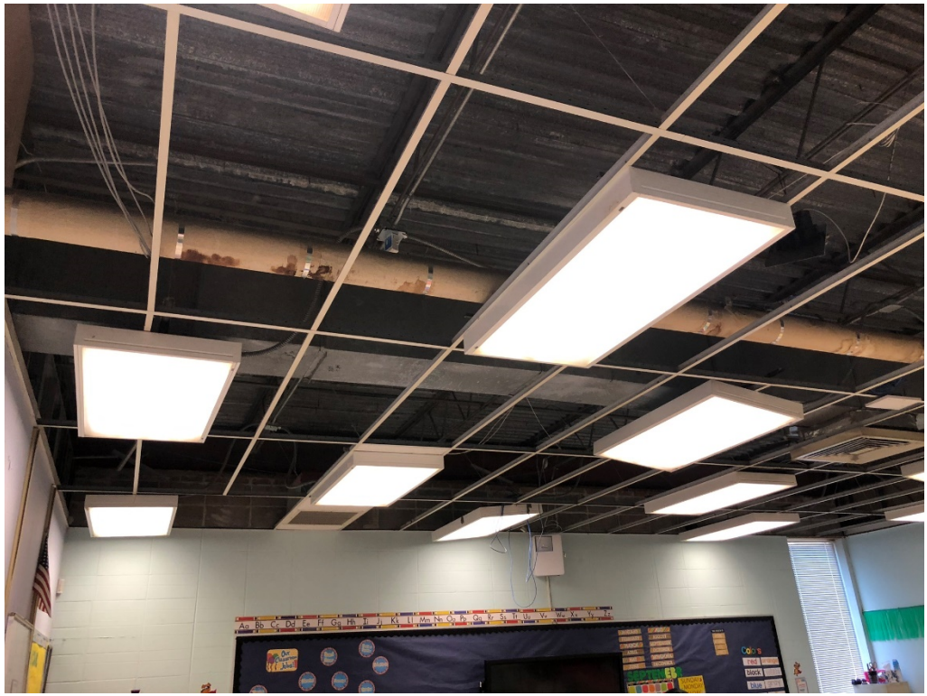
Figure 5 – Power Still Connected for Clients Use of the Room
