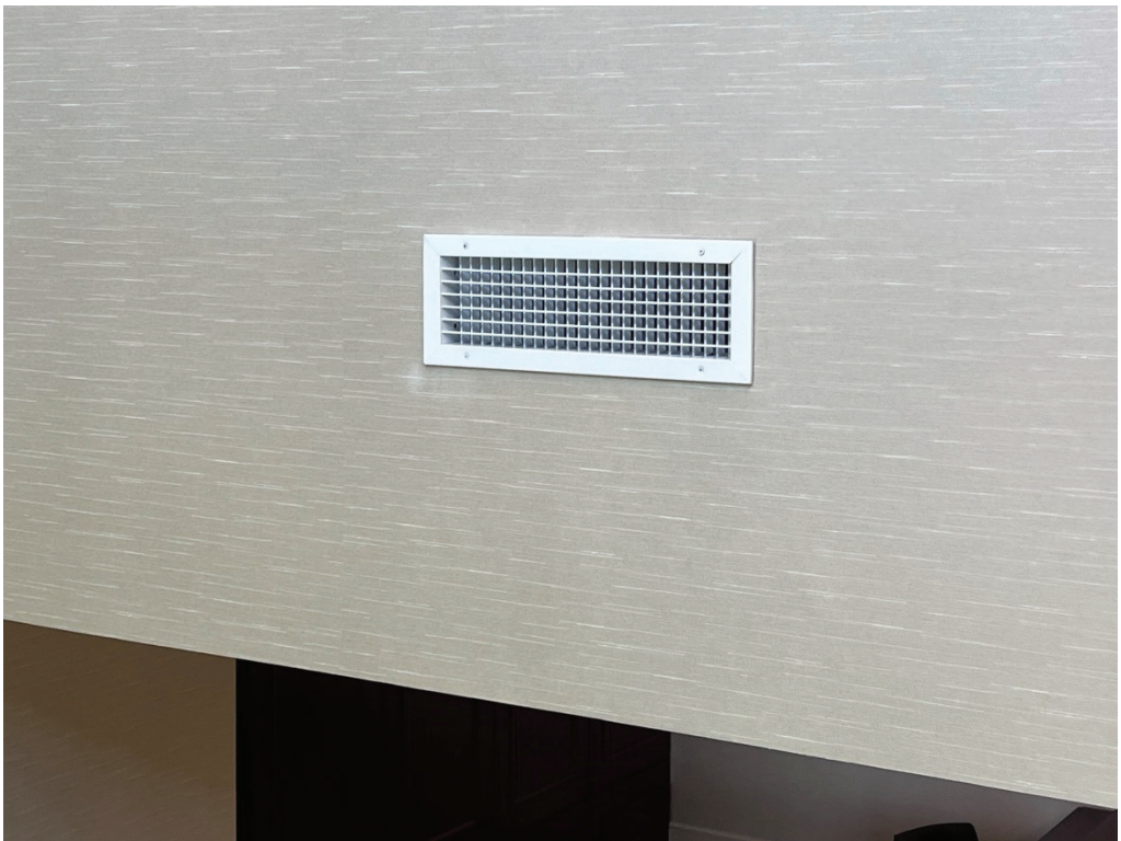
Figure 18 – Some Clean up still needed at vent between 3 rd and 4 th
