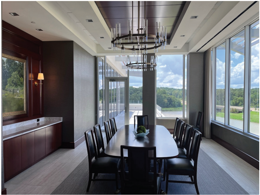
Figure 19 – 4 th Floor Dining with Furniture (still a lot of work needed at ceiling)
