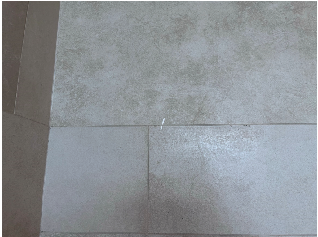
Figure 3 – Paint Noted on Tile Wall in East Lobby
