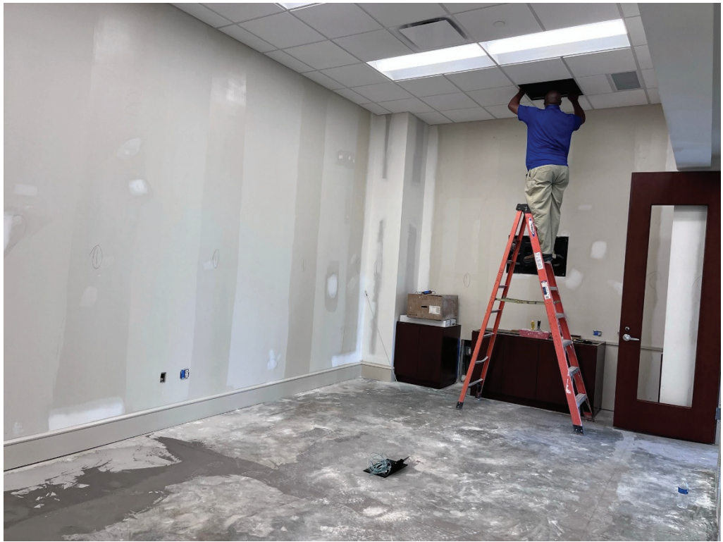
Figure 5 – Network Installer On Site in Conference 1 st Floor
