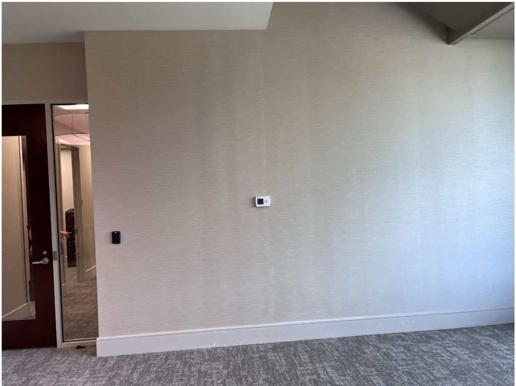
Figure 10 – Repair at 3 rd floor wall still has visible deformities
