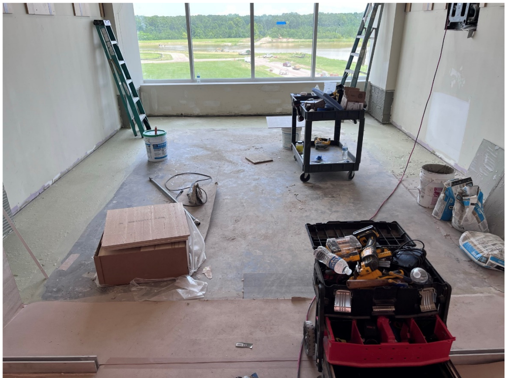
Figure 30 – Tile work has not begun
