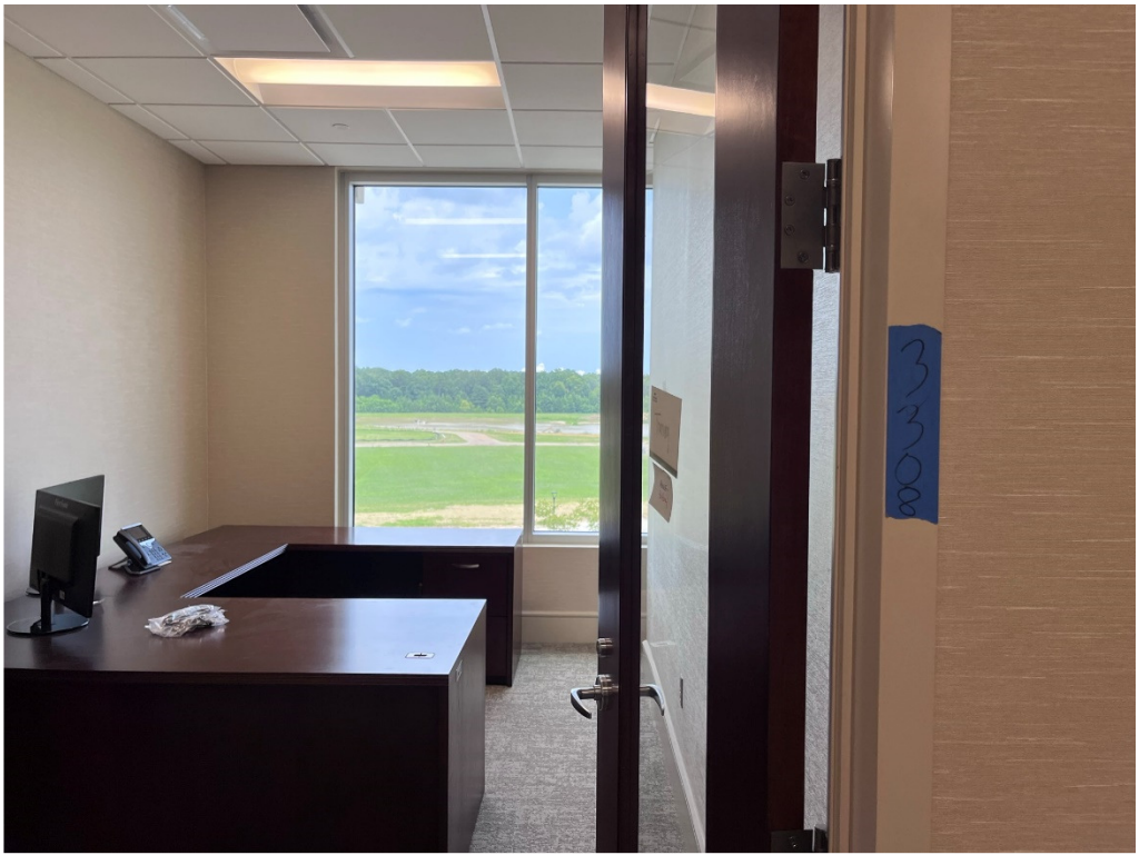
Figure 19 – Room where blinds are missing
