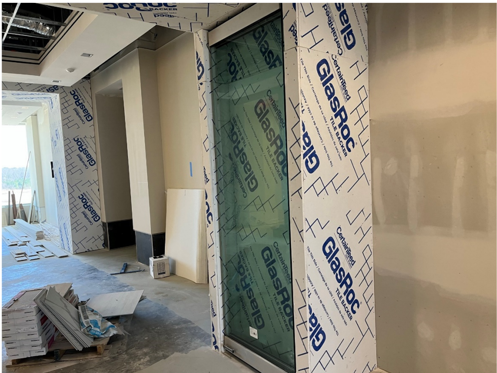
Figure 8 – Doors Recessed per drawings; Owner expressed to contractor prior to install that he wanted glass to be flush with finish tile; these are recessed and will not be flush
