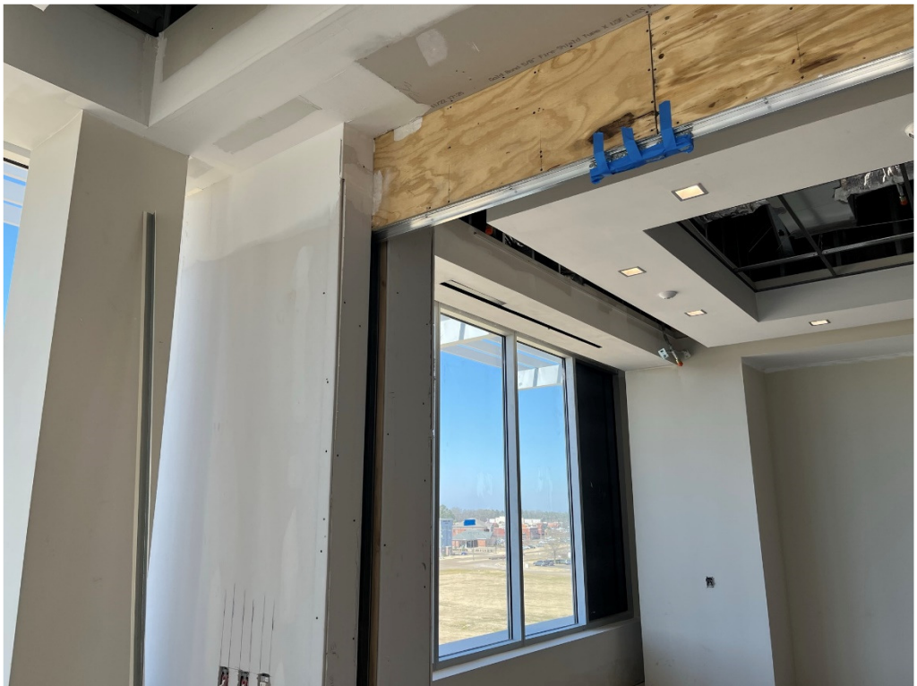
Figure 11 – Sliding Track mounted at Exec Dining
