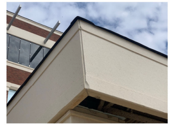
Figure 6 – Corners are not acceptable; missing chipped areas need repair
