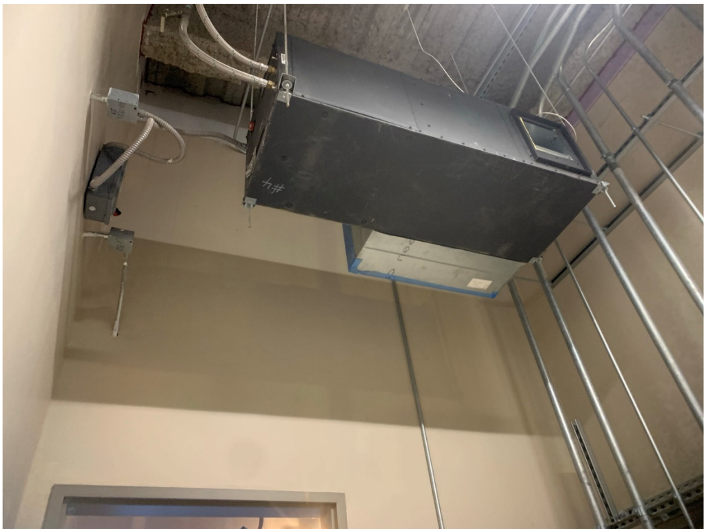
Figure 10 – Unit Missing Drainage
