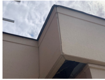
Figure 7 – Corners are not acceptable; missing chipped areas need repair
