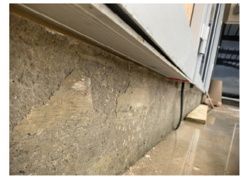
Figure 8 – No Caulking present in some locations below curtain walls assemblies at balconies on 4th
