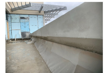
Figure 7 – Bottom edge of new concrete requires straightening at 4 th floor balconies
