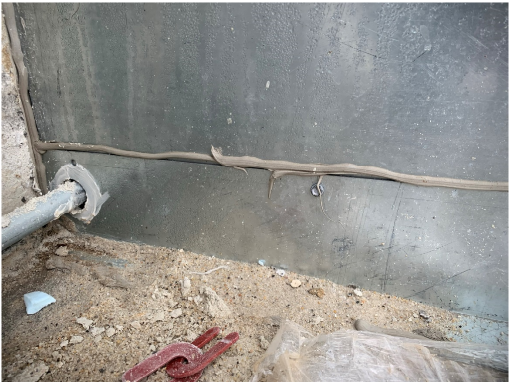
Figure 10 – Poorly caulked flashing will have water intrusion
