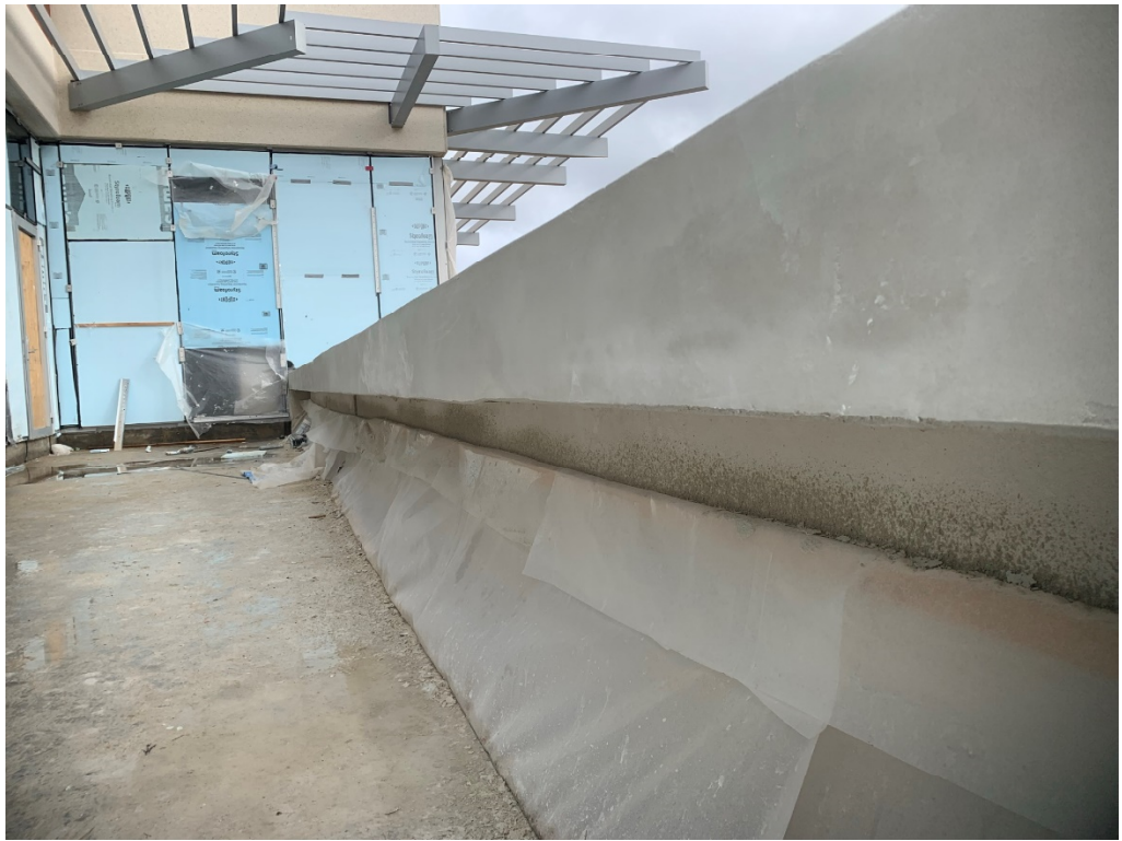
Figure 7 – Bottom edge of new concrete requires straightening at 4 th floor balconies
