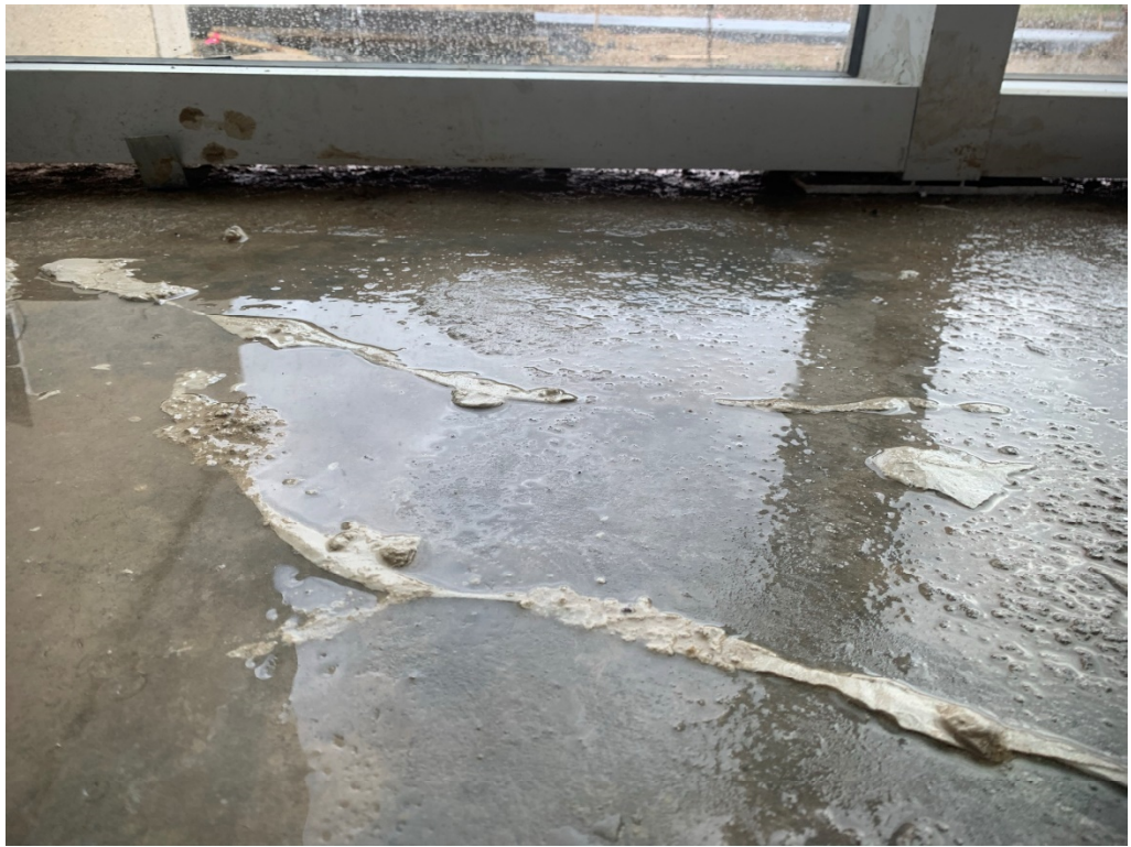
Figure 3 – High moisture levels at the 1 st floor; awaiting elastomeric sealant
