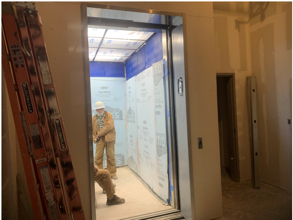
Figure 18 – Maintenance Elevator Operational and in Use
