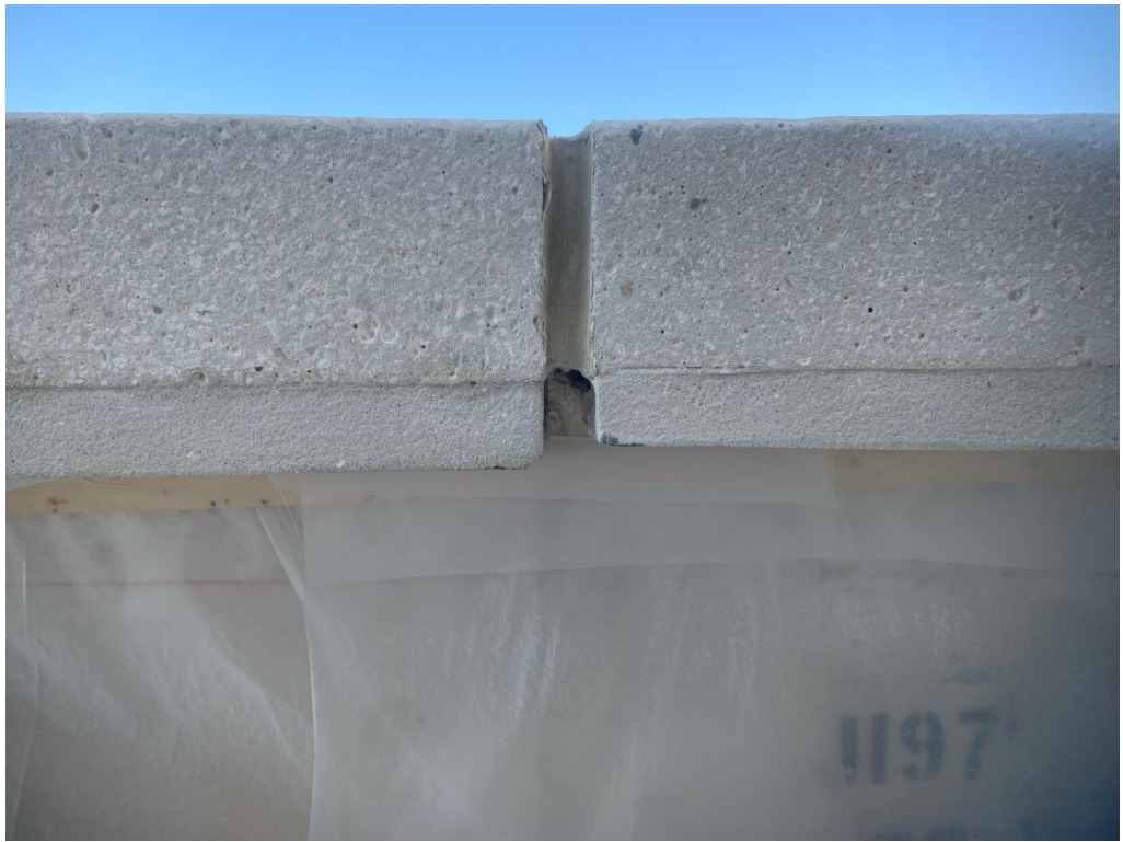
Figure 25 – Mis aligned repair (Is this repair complete or ongoing?)
