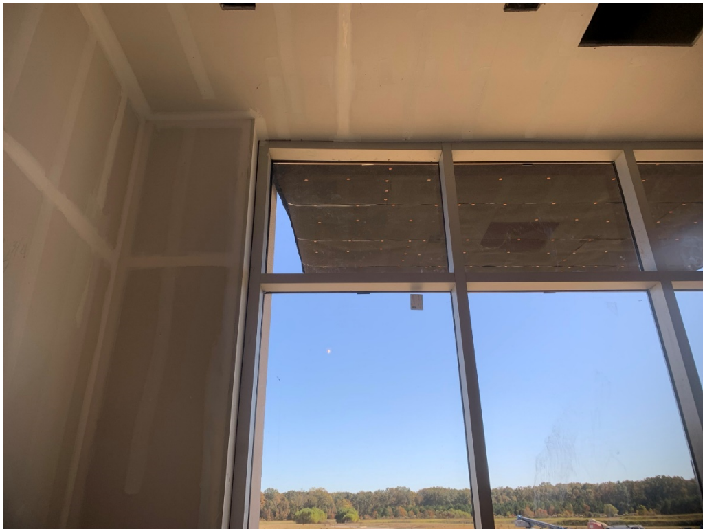
Figure 10 – This opening at column line E is crooked at the top corner
