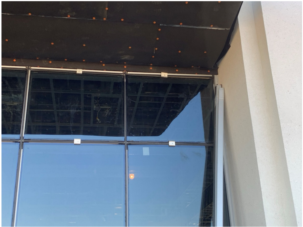
Figure 9 – This opening at column line E is crooked at the top corner
