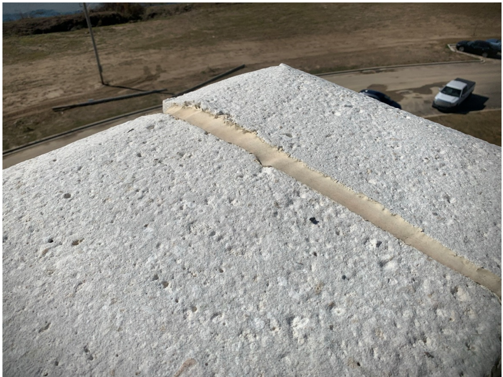
Figure 24 – Are we still awaiting remediation on the sill stones? (these don't line up at the top)
