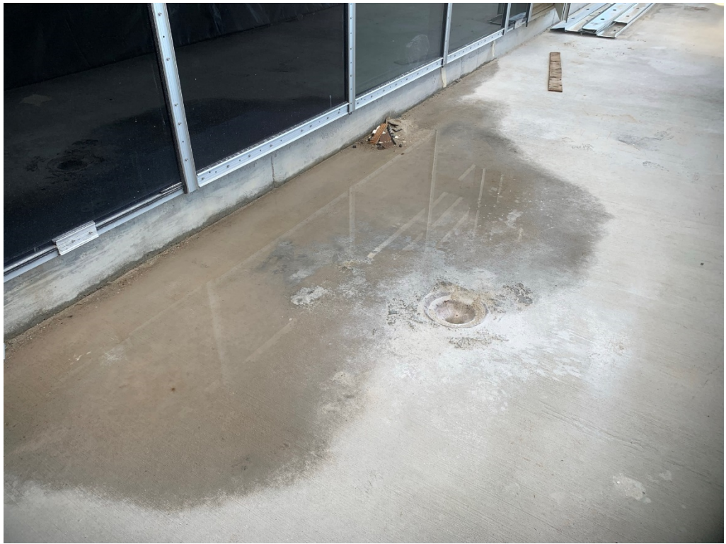
Figure 27 – Pay attention to installation of finish floor so water slopes to drain
