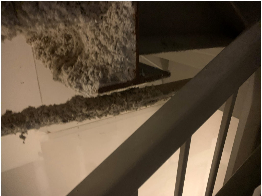
Figure 28 – Can we Chamfer this steel so that it is less threatening? Perhaps this will get worked out in how we're covering the ceilings?
