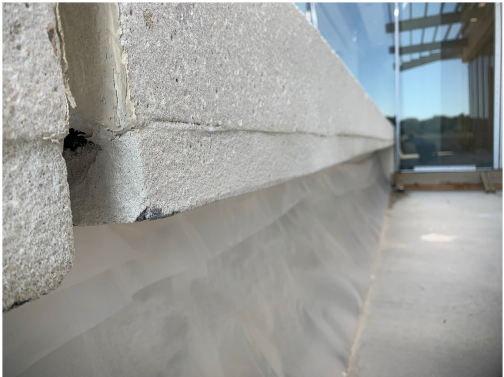
Figure 26 – Mis aligned repair (Is this repair complete or ongoing?)
