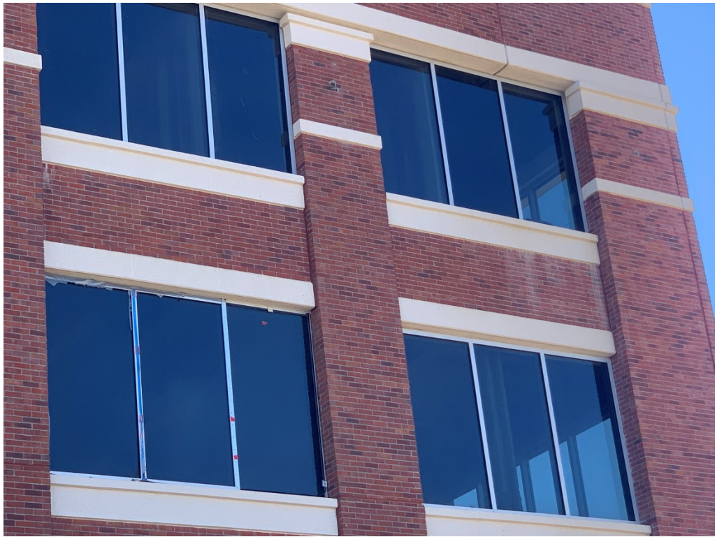
Figure 5 – Effervescence showing at 3 rd story panel when water was received in wall; this will require cleaning; also, have sealant contractor confirm water tightness
