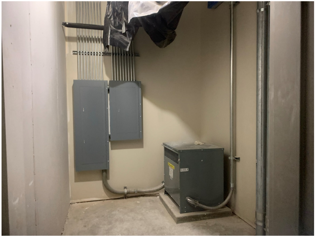
Figure 9 – 2 nd Floor Electrical Room
