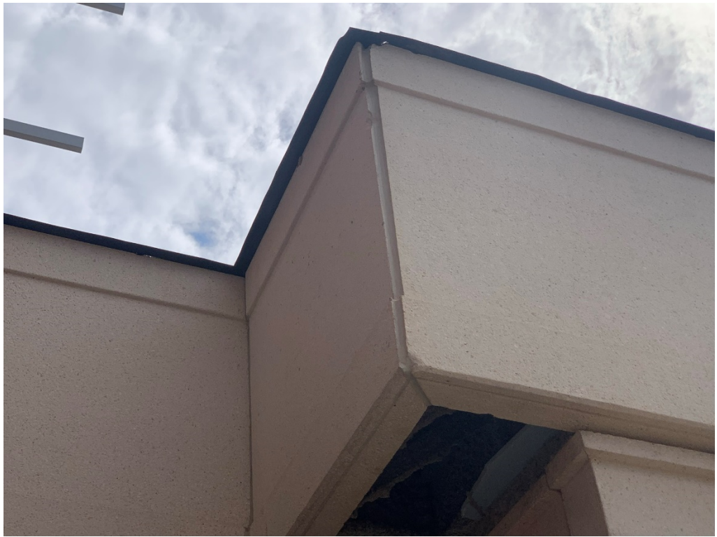
Figure 7 – Corners are not acceptable; missing chipped areas need repair
