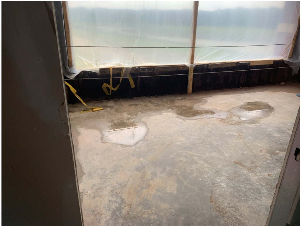
Figure 11 – Water Intrusion is ongoing
