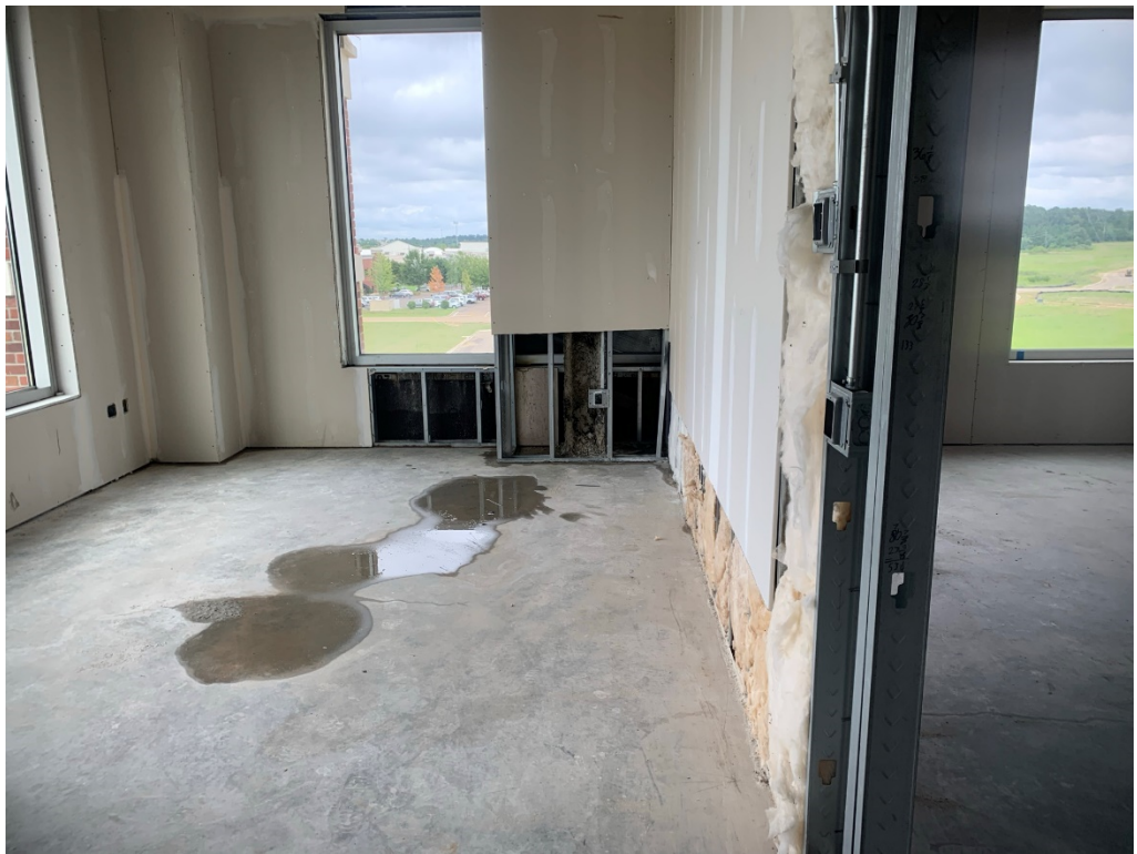
Figure 12 – Water Intrusion is ongoing
