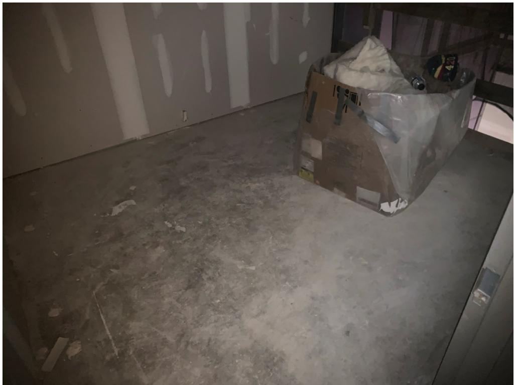
Figure 10 – Support 2007: this floor seems to be very out of level and may need additional leveling installed at the floor
