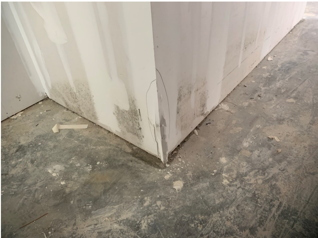
Figure 12 – Interior Walls should be cut 24" from floor wherever mold has set in and insulation removed for drying
