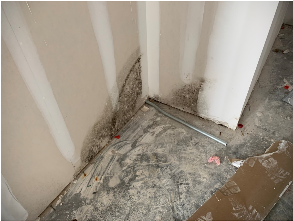
Figure 11 – Interior Walls should be cut 24" from floor wherever mold has set in and insulation removed for drying
