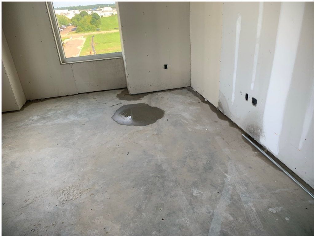
Figure 10 – This NW 3 rd Floor Corner Office should have all sheetrock removed and insulation for drying
