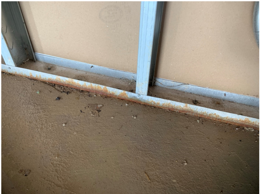
Figure 8 – This is evidence of significant rust at the first floor walls; bottom plate should be replaced after project is dried in.
