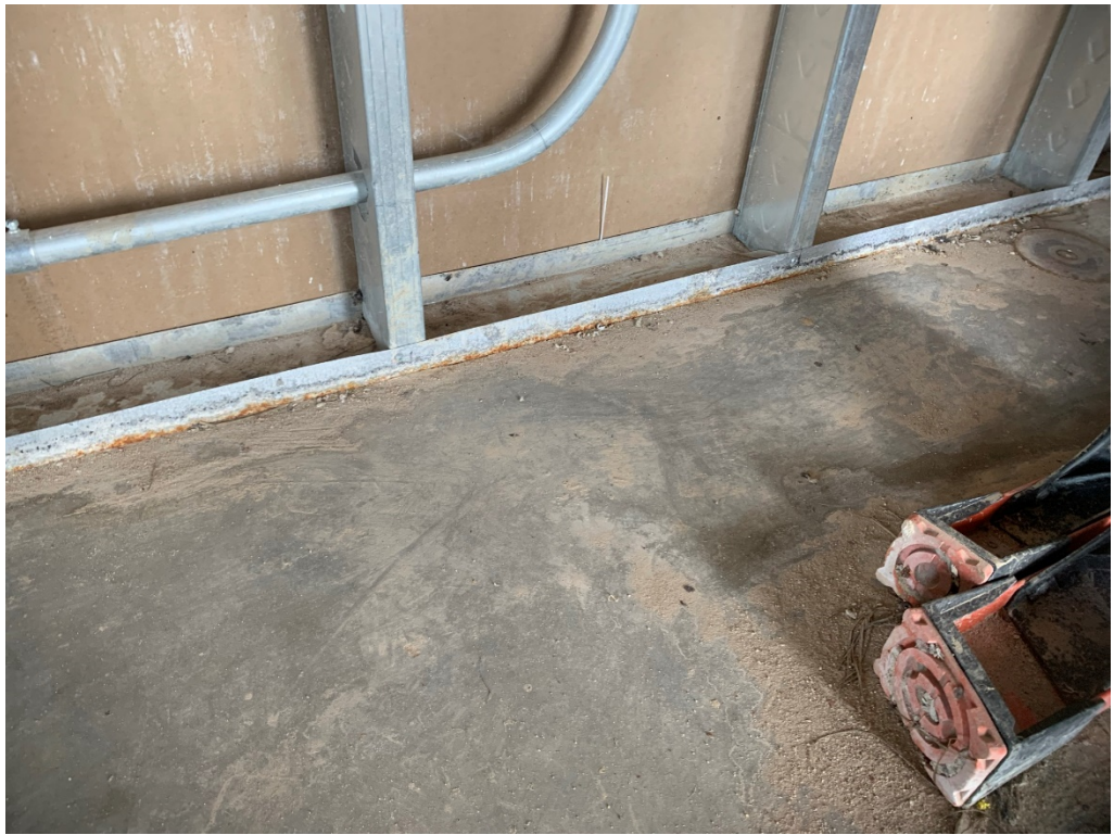
Figure 7 – This is evidence of significant rust at the first floor walls; bottom plate should be replaced after project is dried in.
