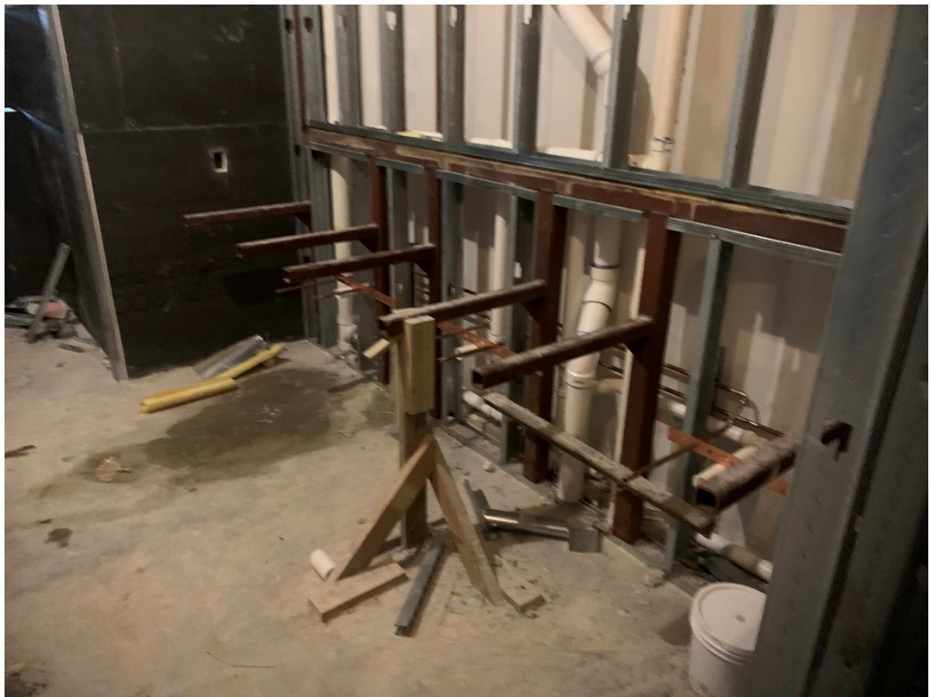
Figure 12 – 2 nd Floor Bathroom Carriers
