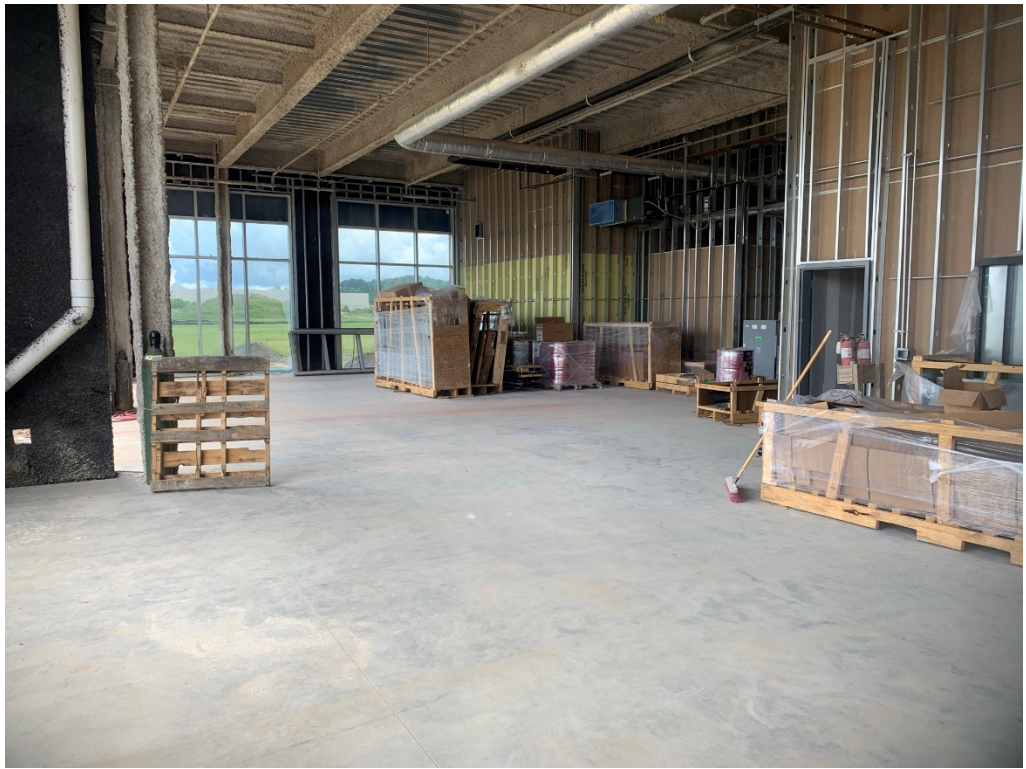
Figure 3 – Swept 1 st Floor; Elevator Parts Stored Here
