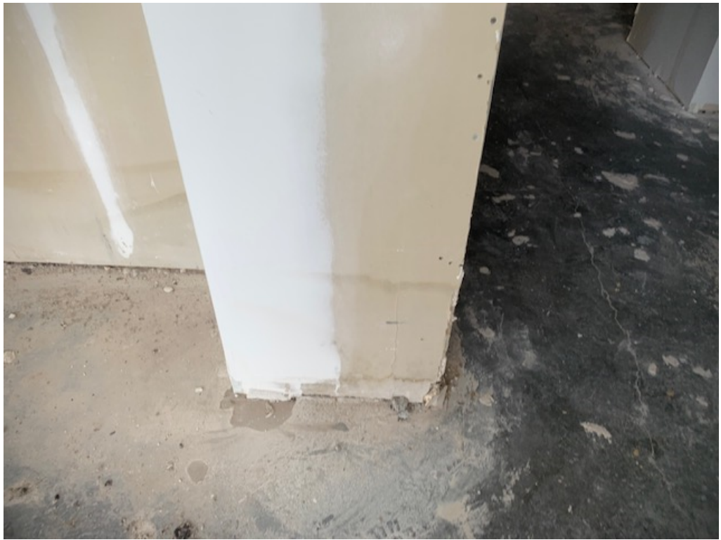
Figure 9 – Water Damaged Drywall Should be Replaced (noted primarily at 3 rd floor SE)
