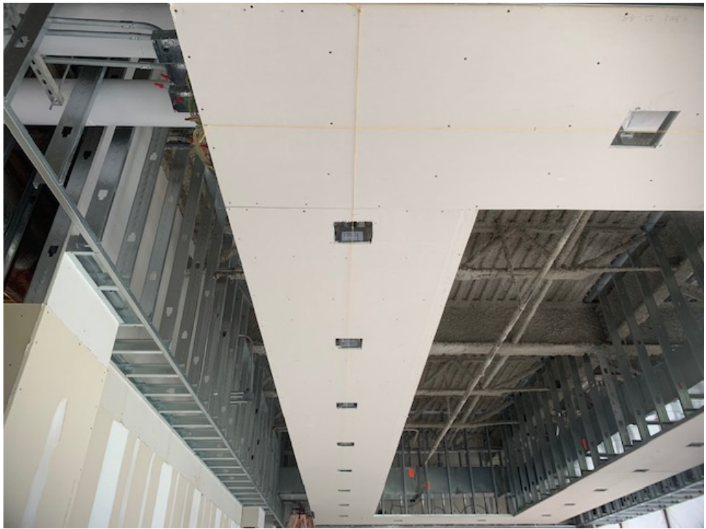
Figure 17 – Ceiling Lighting at Board Room
