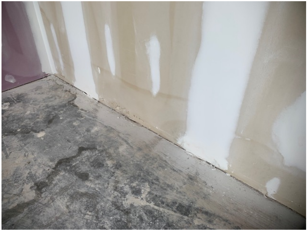
Figure 11 – Water Damaged Drywall Should be Replaced (noted primarily at 3 rd floor SE)
