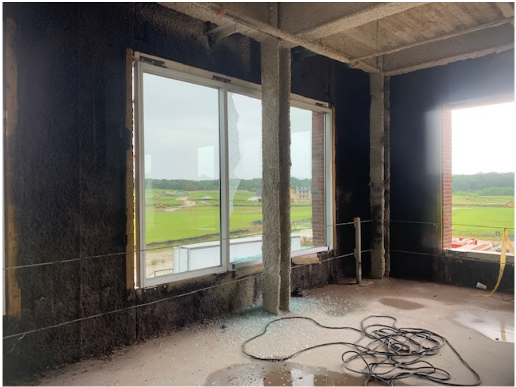
Figure 7 – Broken Glass at 2 nd Floor North Windows
