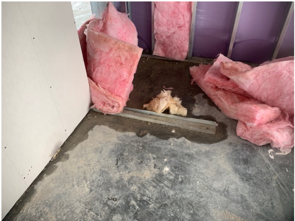
Figure 14 – Wet Insulation should be Discarded and Replaced
