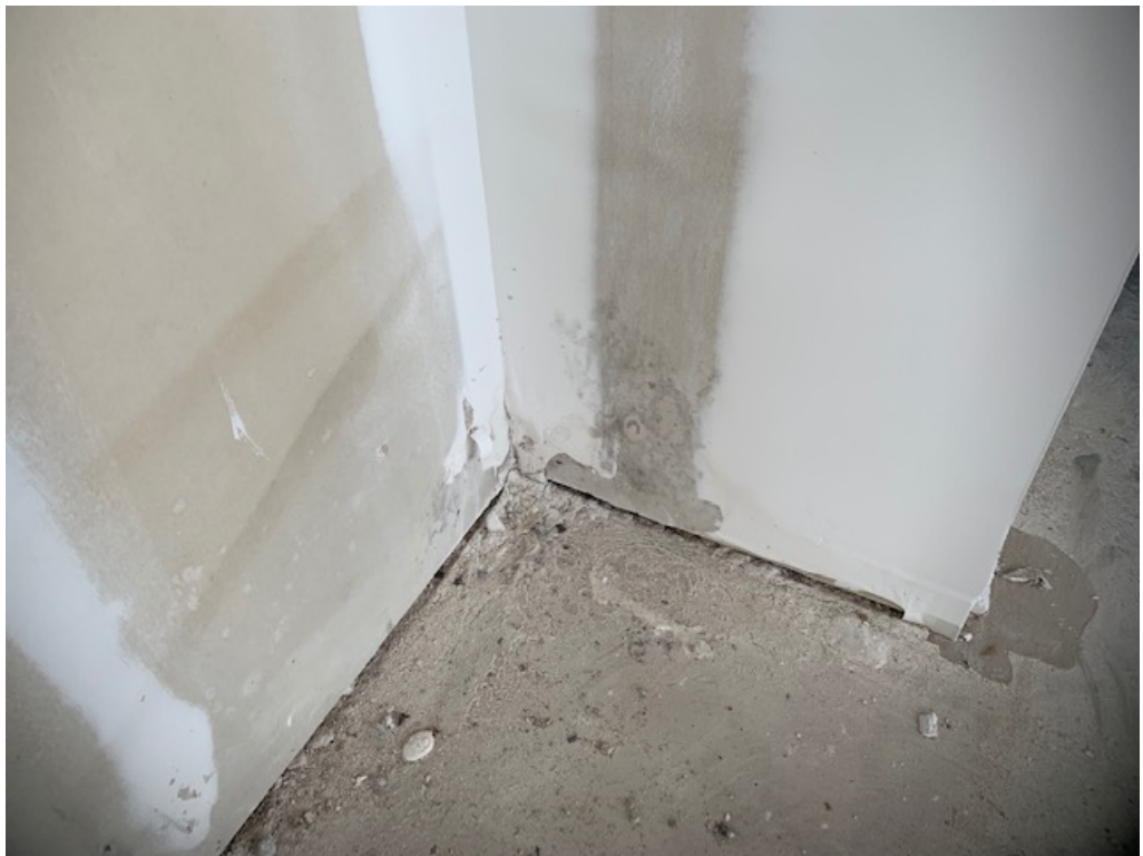
Figure 10 – Water Damaged Drywall Should be Replaced (noted primarily at 3 rd floor SE)
