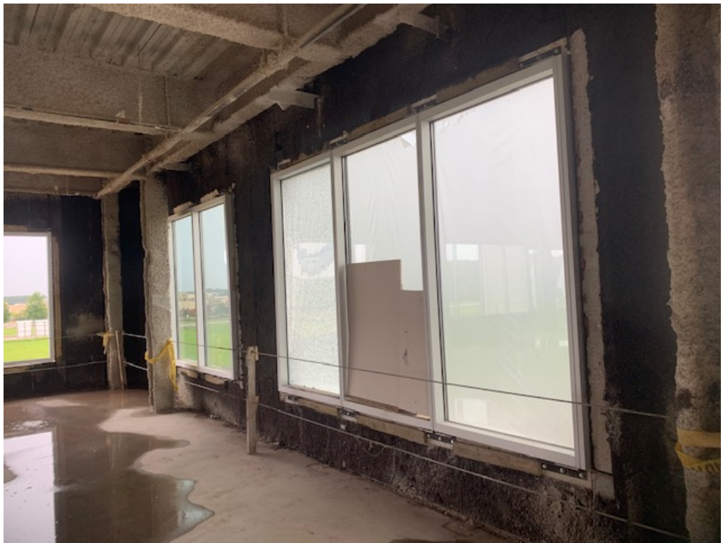
Figure 6 – Broken Glass at 2 nd Floor North Windows
