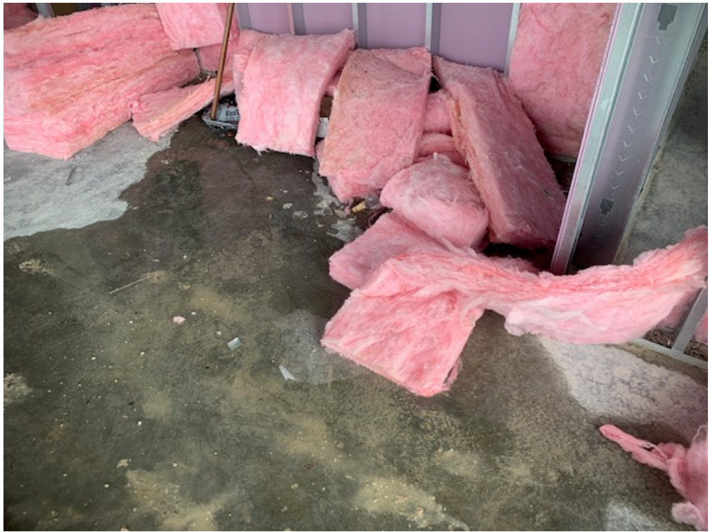
Figure 15 – Wet Insulation should be Discarded and Replaced
