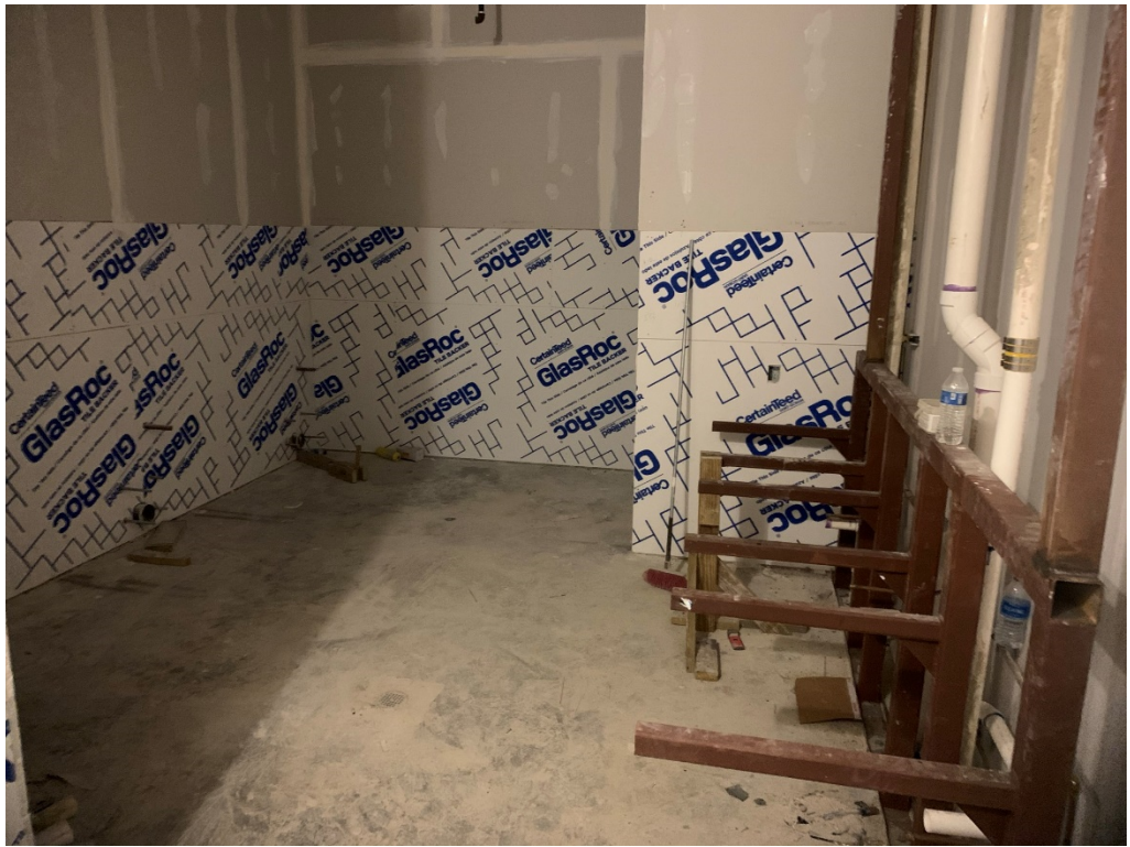
Figure 9 – Carriers installed at 4004
