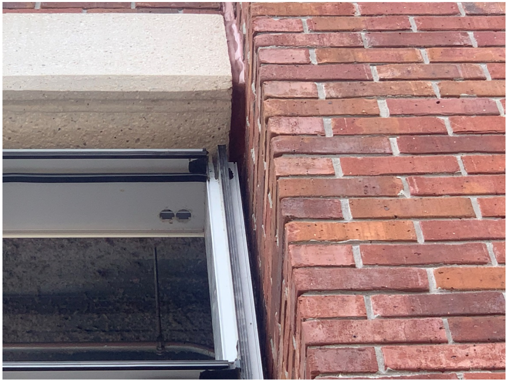
Figure 15 – Typical Gaps between curtain Wall and Panels (per manufacturer joints between ½" to 1" require ½" depth of sealant; over 1" require regional service consultation)
