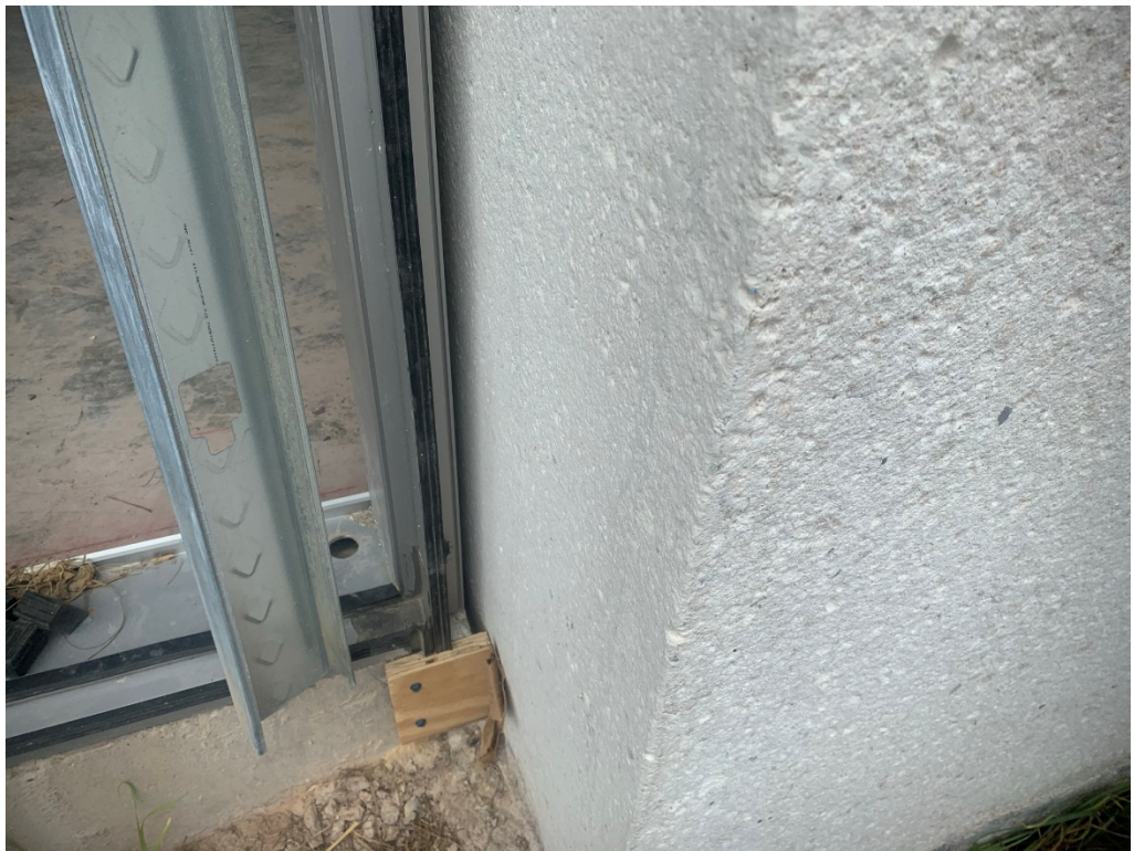
Figure 14 – Typical Gaps between curtain Wall and Panels (per manufacturer joints between \frac{1}{2} " to 1" require \frac{1}{2} " depth of sealant; over 1" require regional service consultation)
