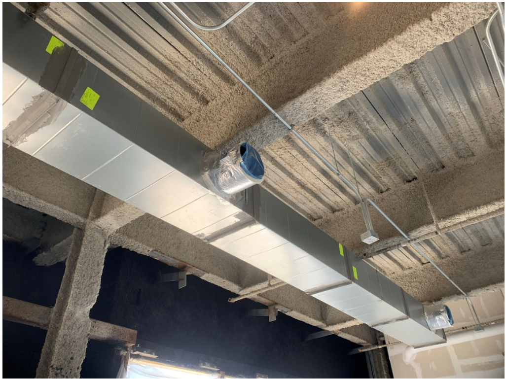
Figure 7 – Uncovered Ducting at 4 th Floor
