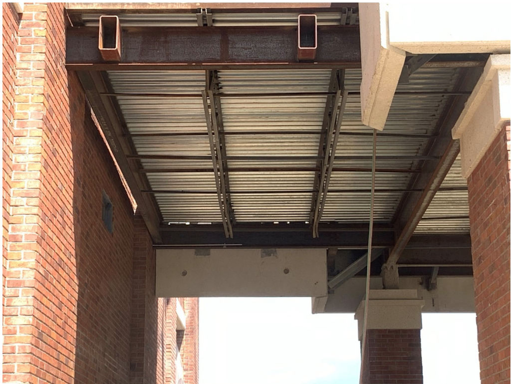
Figure 2 – Open Web joists Damaged and need straightening or replacement
