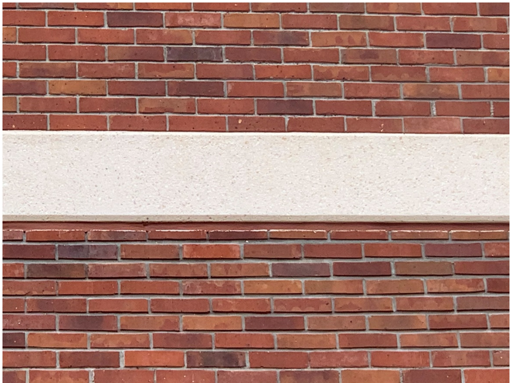
Figure 6 – White Caulk, previously installed, needs removal
