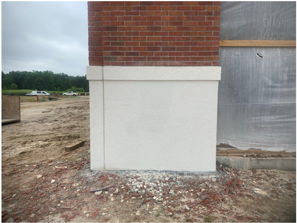
Figure 7 – Shade still showing through finished panel
