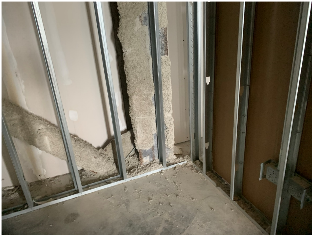
Figure 12 – Fire Insulation Still Missing in Areas
