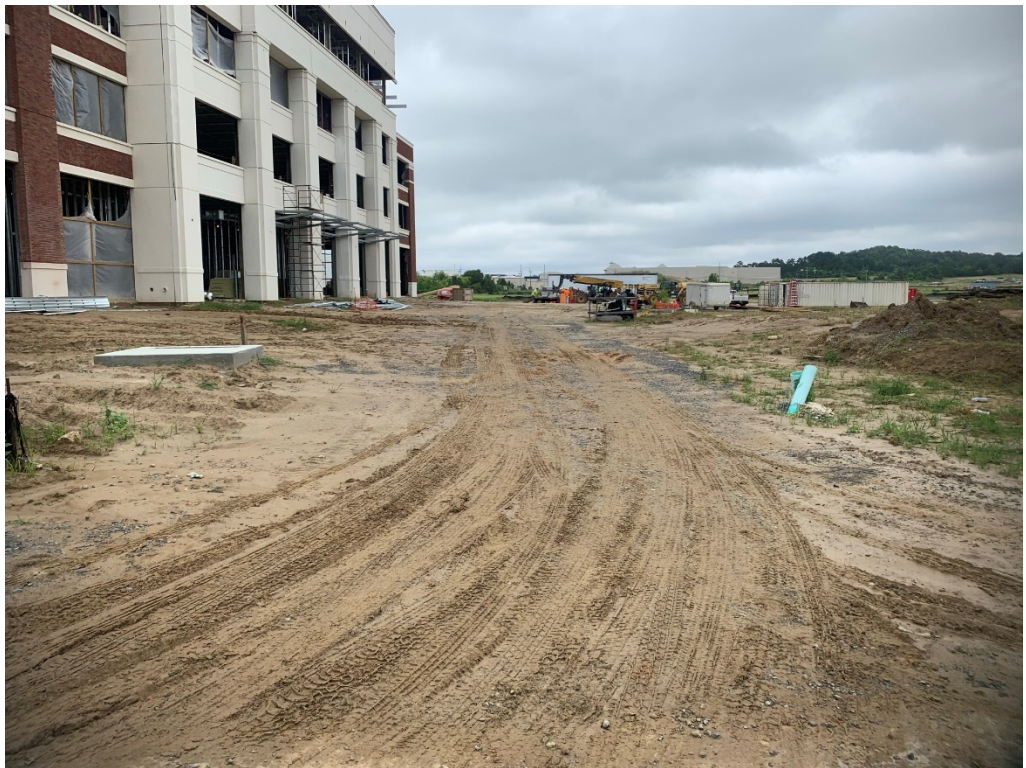
Figure 2 – Concrete Pad is approximately 25' from markers on right
