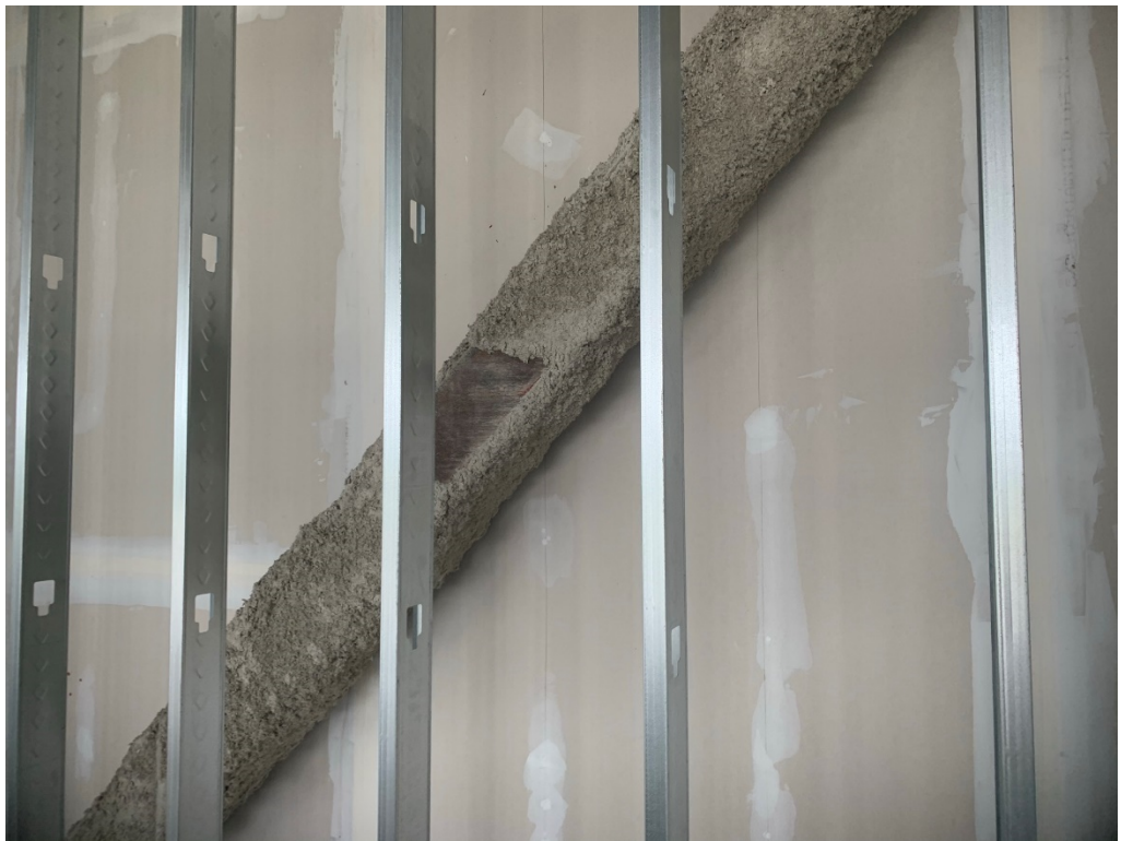
Figure 16 – Fire Insulation Needs Repair
