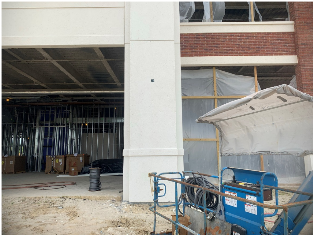
Figure 4 – Recessed edge on right has been colored and is different than the other faces
