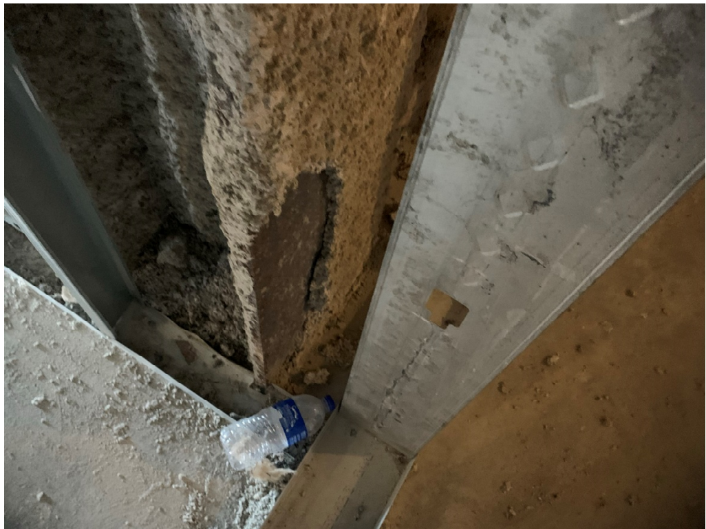
Figure 14 – Fire Insulation Needs Repair
