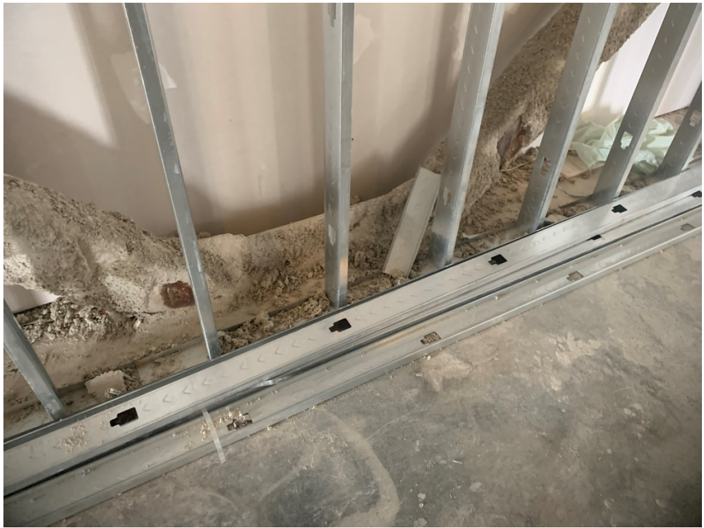
Figure 15 – Fire Insulation Needs Repair
