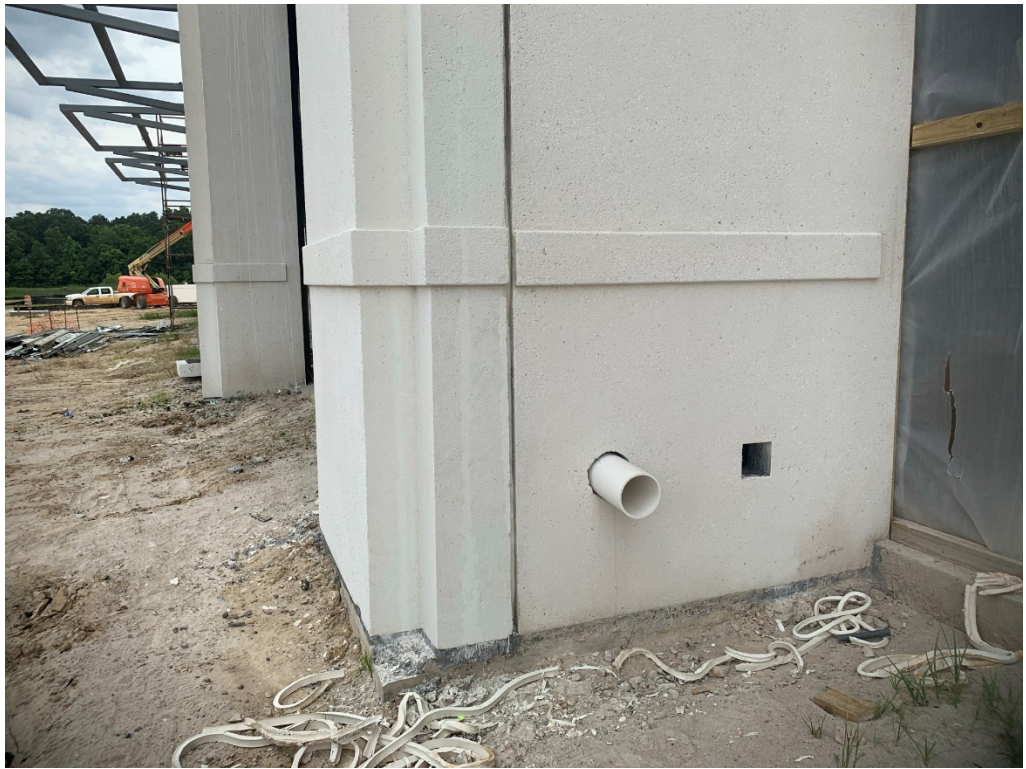
Figure 3 – Repair at Column after 5 days of cure time still not blending
