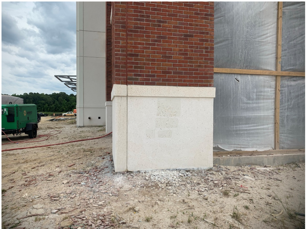
Figure 2 – Repair at Column after 5 days of cure time still not blending
