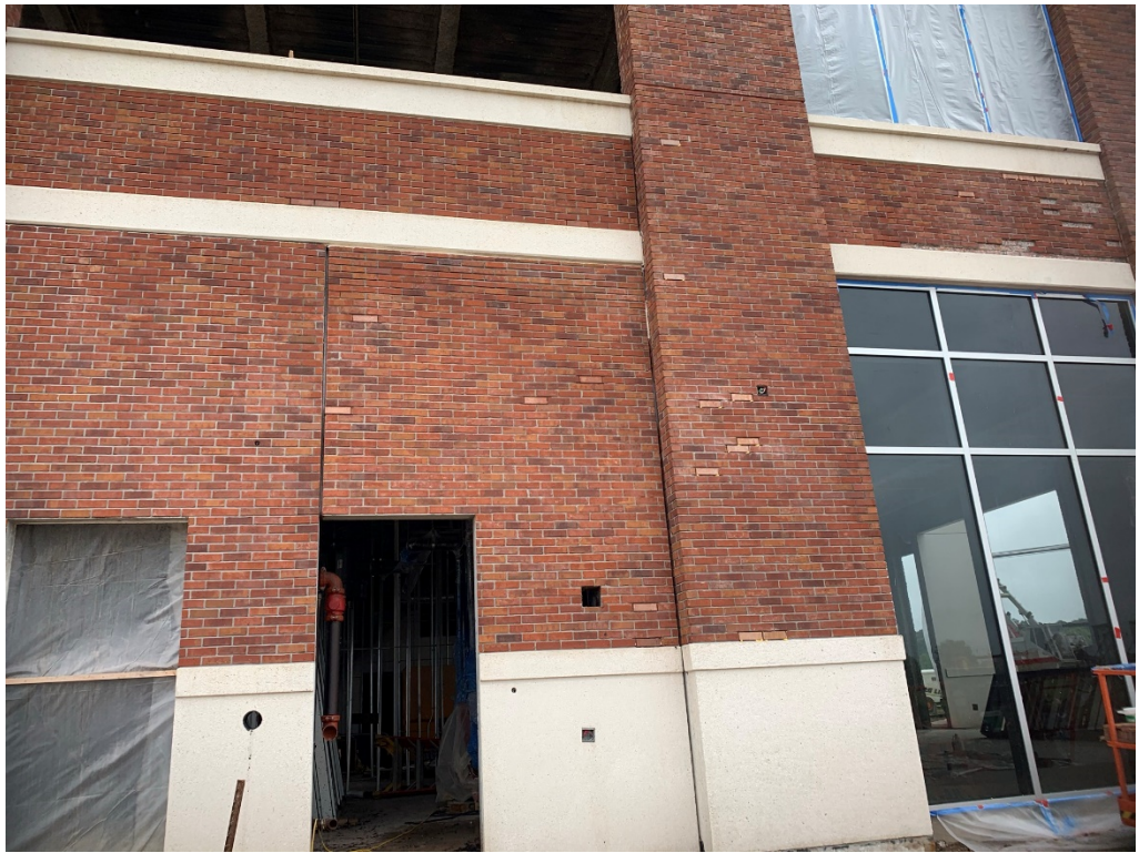
Figure 3 – Sealant Progress Stalled due to Shortage of Material and Rain
