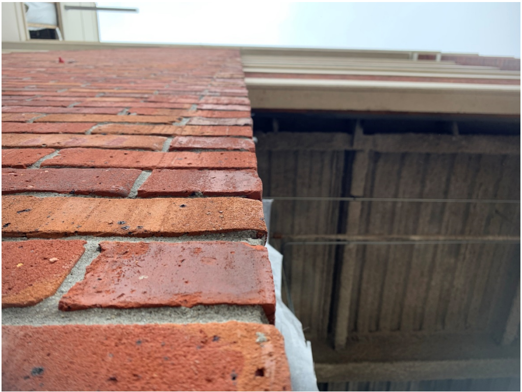
Figure 1 – Brick Corner at Repaired Panel at Front Elevation
