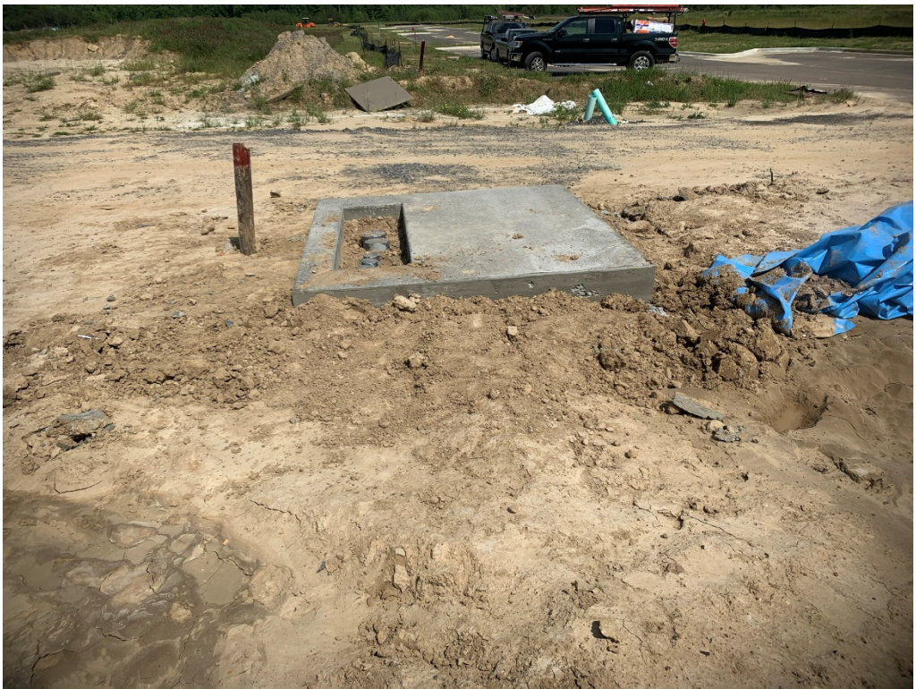
Figure 6 – Electrical Conduit to Transformer installed
