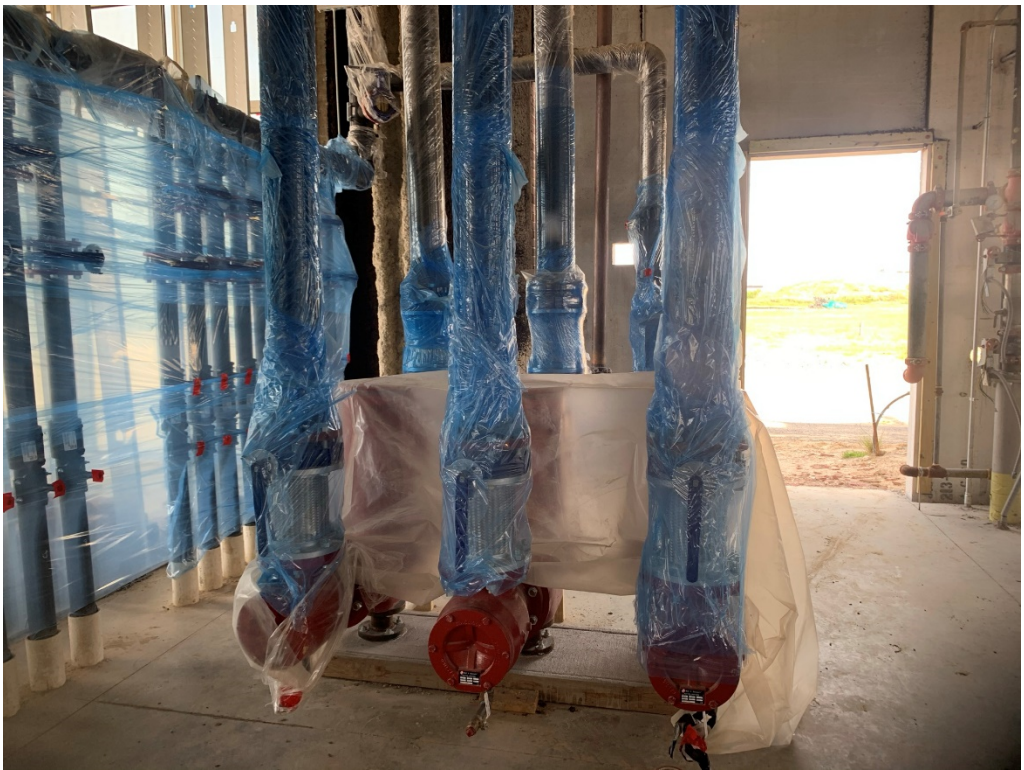
Figure 12 – Sprinkler Risers Protected
