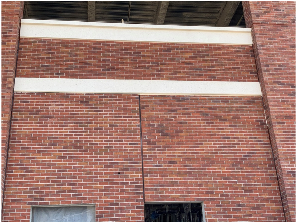
Figure 3 – Sealant Progress Stalled due to Shortage of Material
