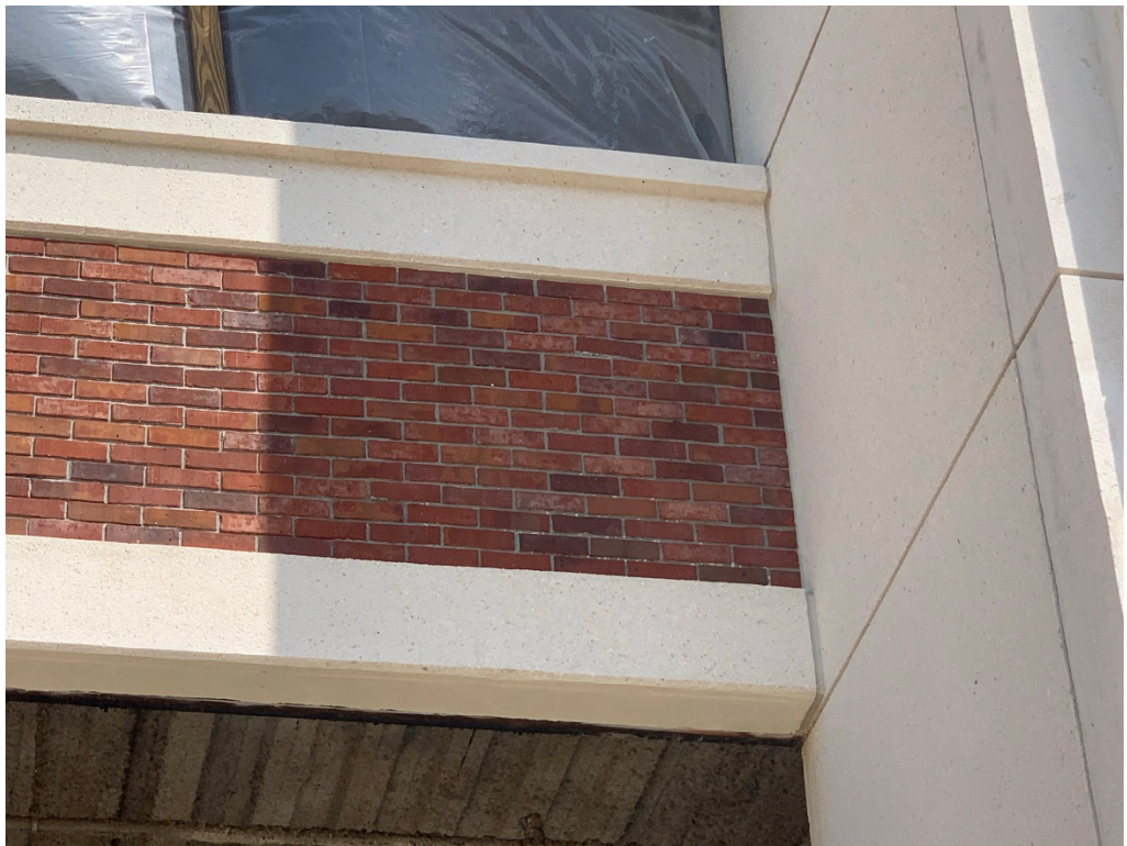
Figure 2 – White Sealant here looks good
