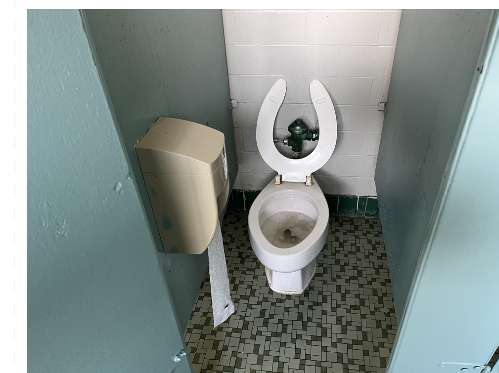
Typical Toilet Style
