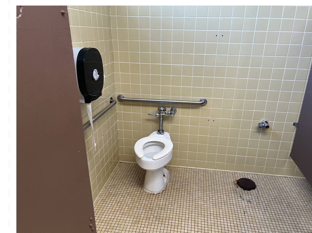
Typical Toilet Style
