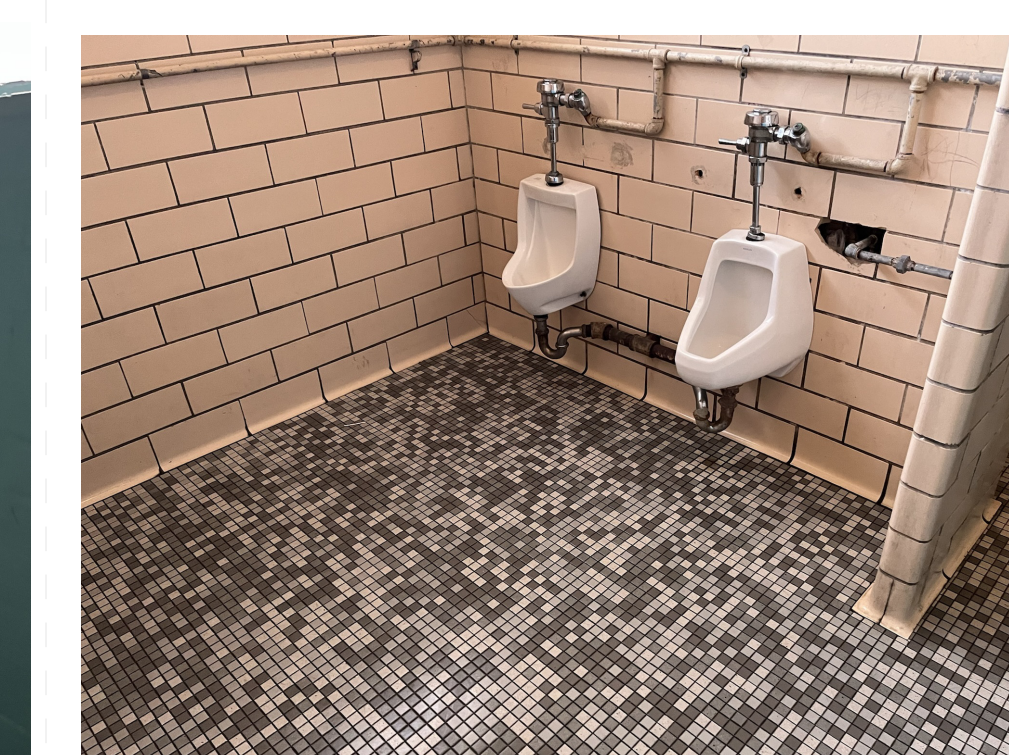
Middle Bldg Urinals
