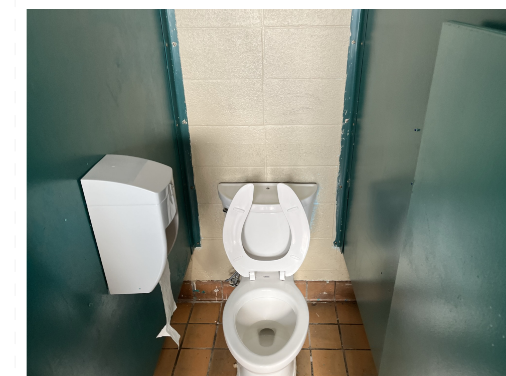
Typical Toilet Style
