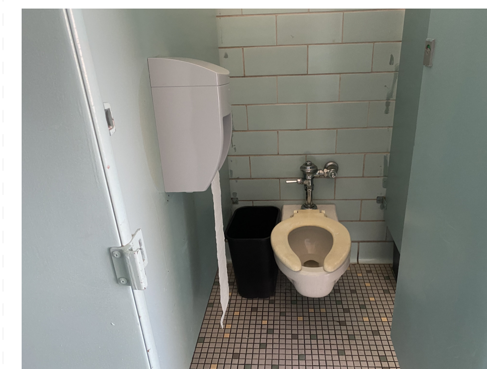
Typical Toilet Style
