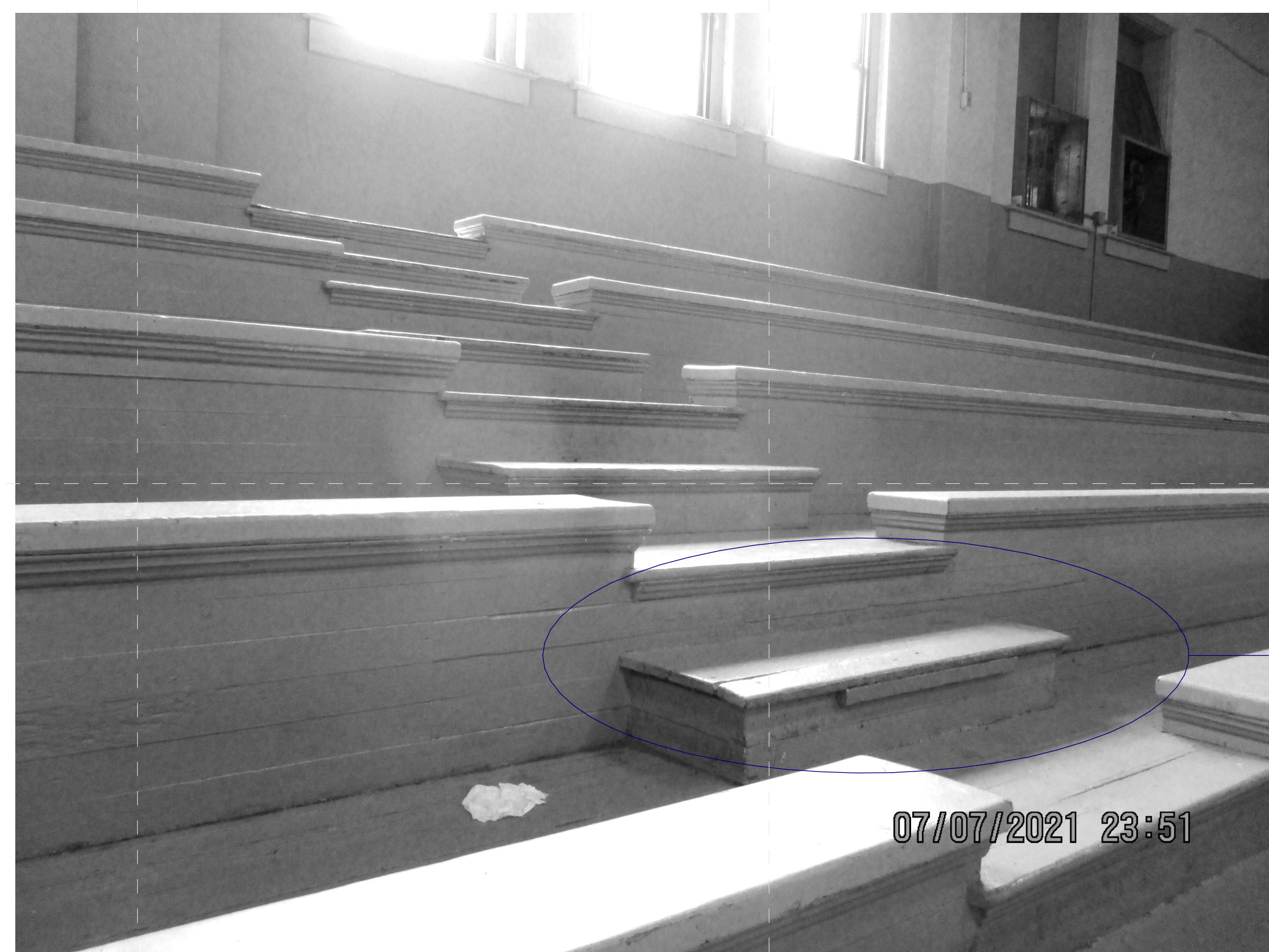
Example of Typical Repair
