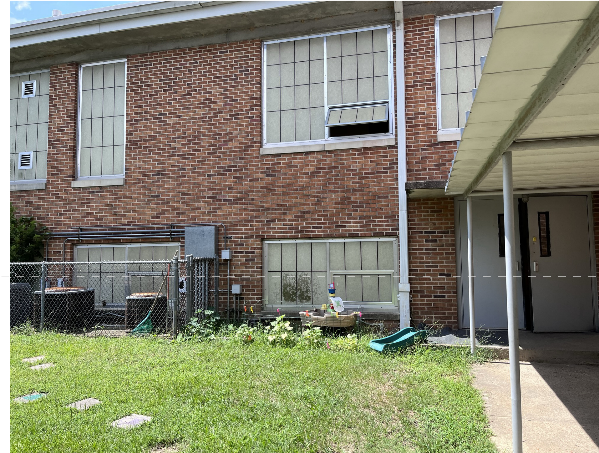
Typical Double Doors to be Replaced
