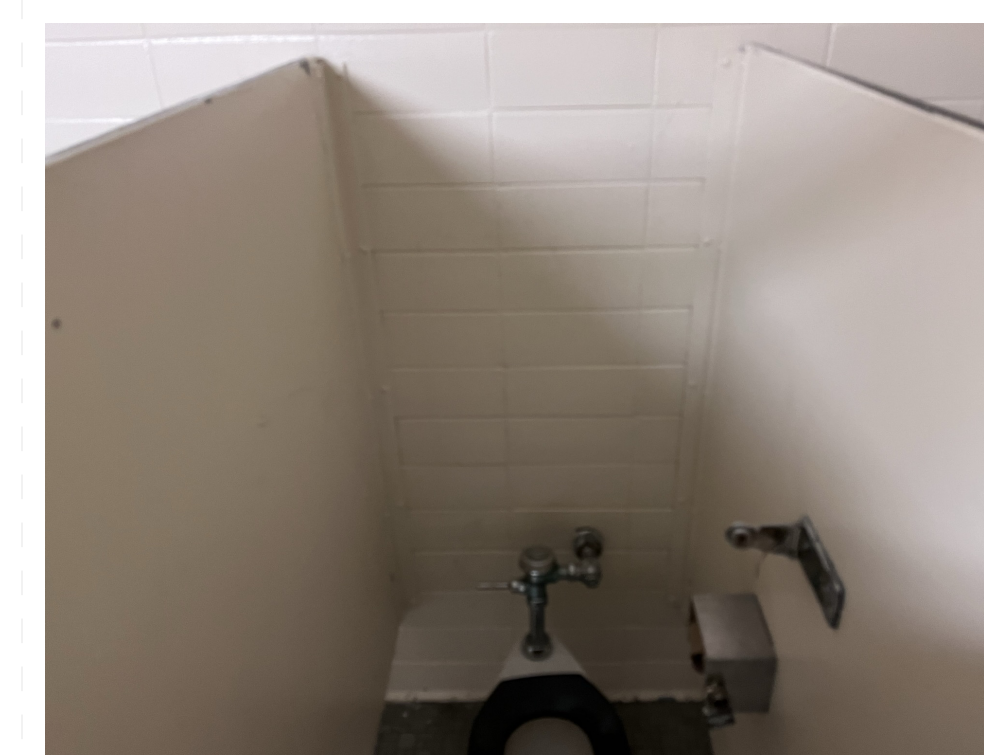
Typical Toilet Style
