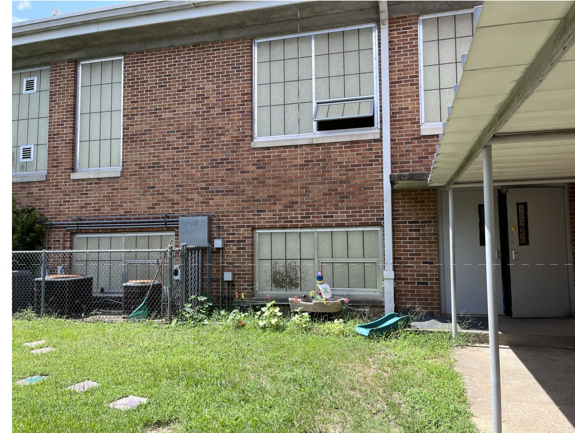
Typical Double Doors to be Replaced
