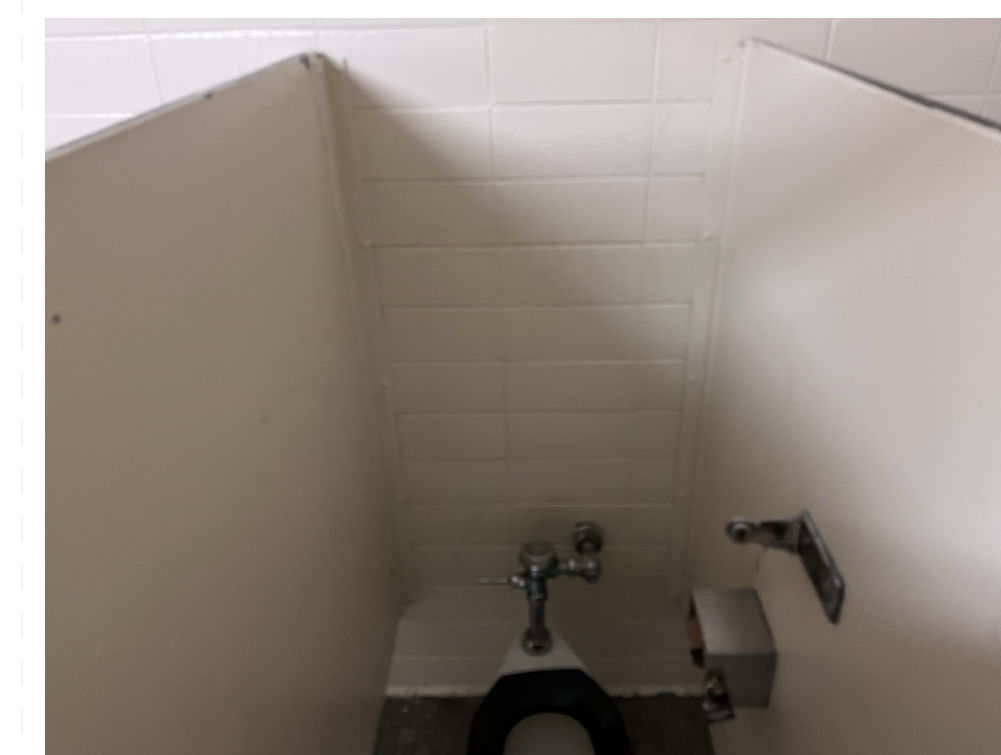
Typical Toilet Style
