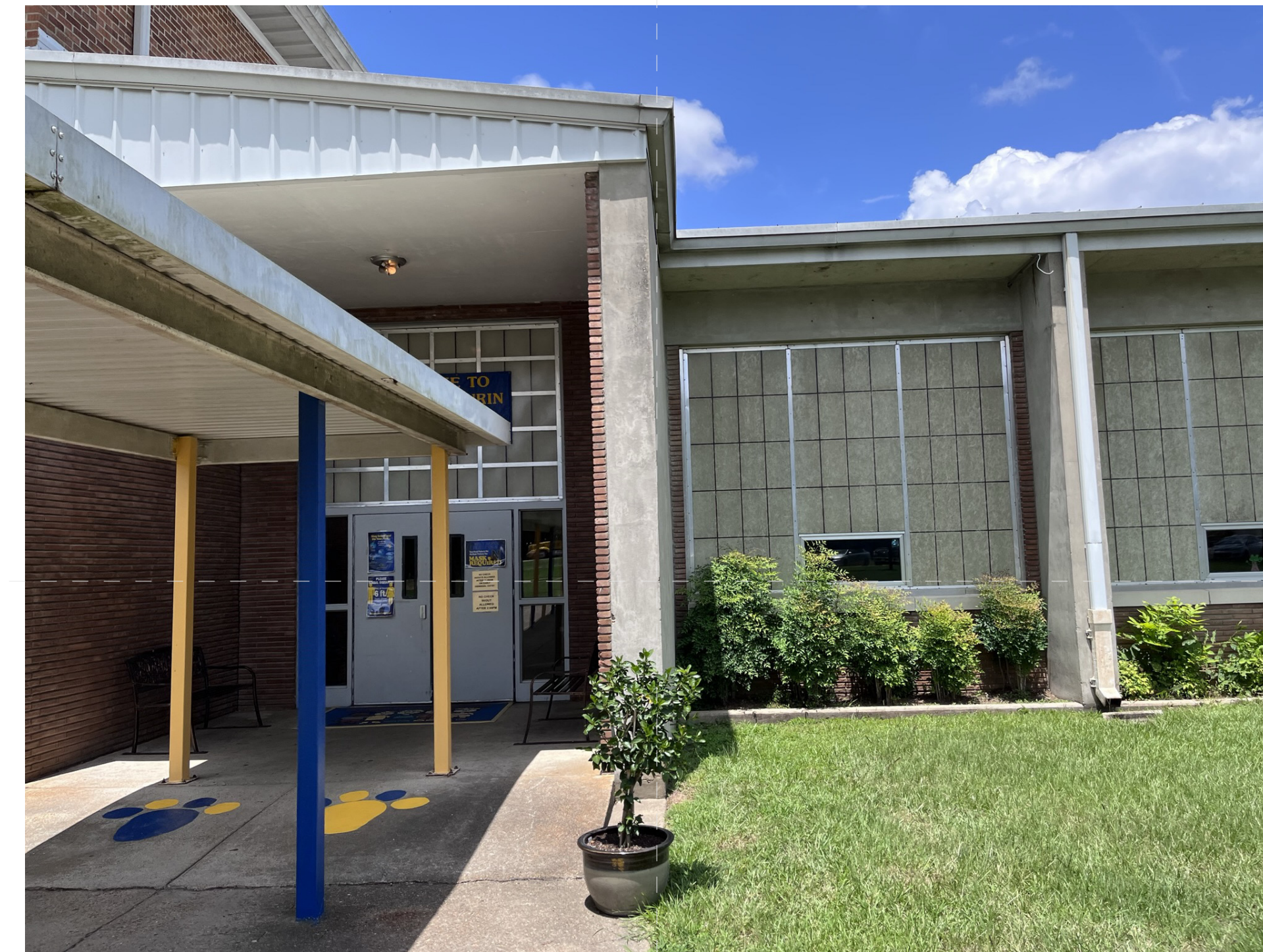
Entry Double Doors to be Replaced
